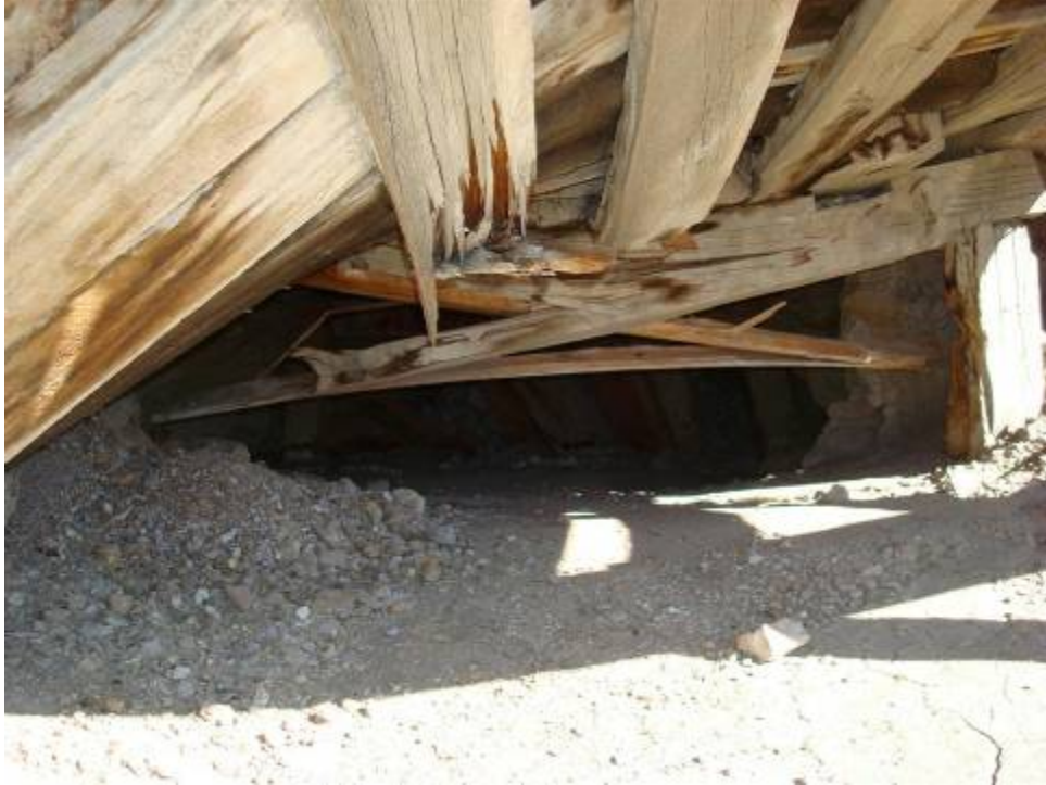
Photo 5. Alta Mine site, collapsed adit
