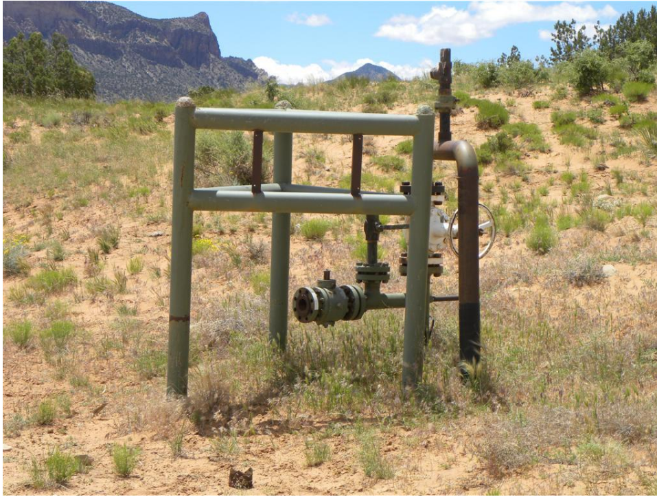
Photo 5. Plot 1 site, piping running through site
