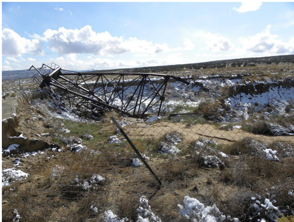
Photo 10. Fallen tower at mine site south of Isabella
