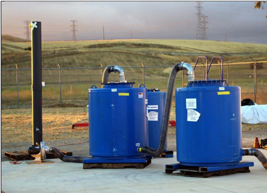
Figure 13. Activated carbon scrubber system installed on the railcar
