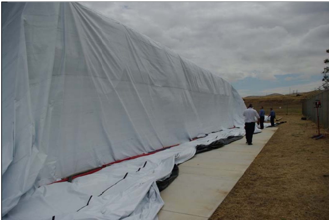
Figure 3. Skirt of EVOH tarp dropped to the ground and weighed down with sandbag “snakes”
