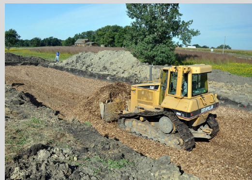
Installing a denitrifying bioreactor in a Midwest field. Photo by J. Johnson, USDA NRCS.
