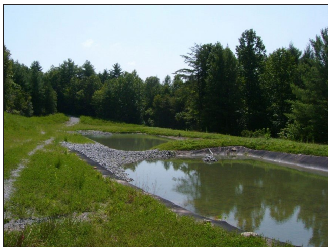
Figure 1. One of eight acid mine drainage treatment ponds installed in the Crab Orchard Creek watershed.
