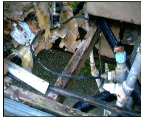
Photograph depicting the rotted floors of MHU2. The floor cavities were exposed raising a safety concern
