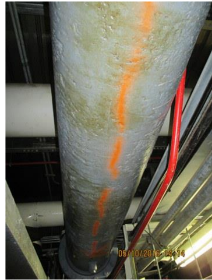
Figure 1. Example of Pitting on Pipeline in Lower Access Tunnel
