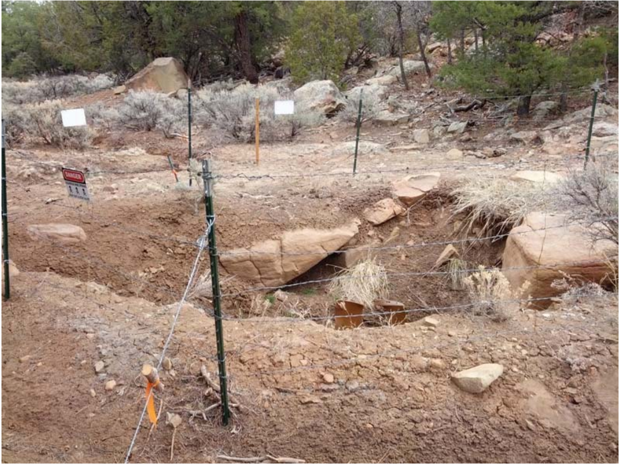
PHOTO 5: Ruby Mine #1 Vent fencing and warning signage, facing northeast.
