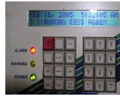
ATG in alarm status
