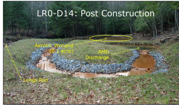
Figure 3. At site LR0-D14, AMD flows through an open limestone channel passive treatment system and into a small aerobic wetland before discharging to Longs Run.
