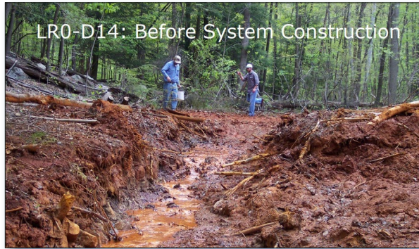
Figure 2. Before project implementation, AMD flows emerging from a seep in the hillside caused erosion and carried pollutants. (Photos by Skelly and Loy, Inc.)
