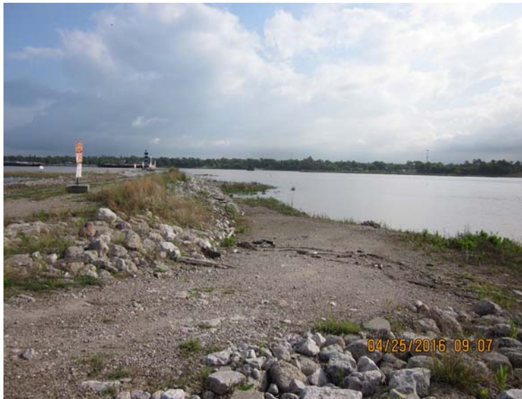
Photograph 19: Central berm after heavy rainfall the week of April 18, 2016 (view north)
