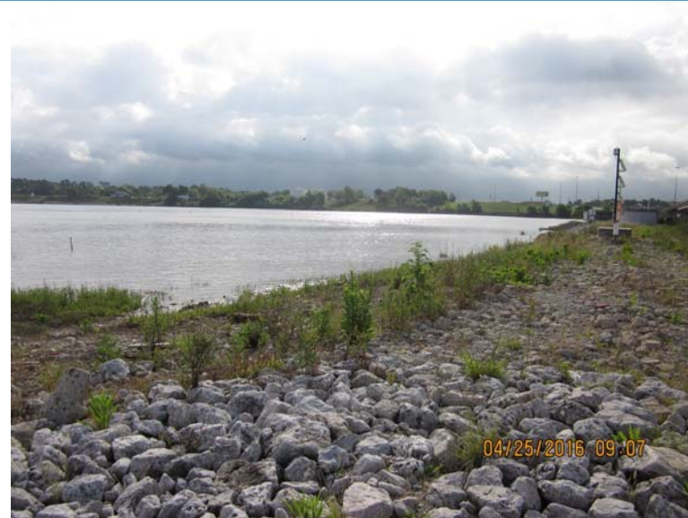
Photograph 18: Southern berm after heavy rainfall the week of April 18, 2016 (view northeast)
