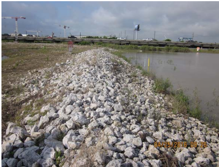
Photograph 23: Western berm after heavy rainfall the week of April 18, 2016 (view south)
