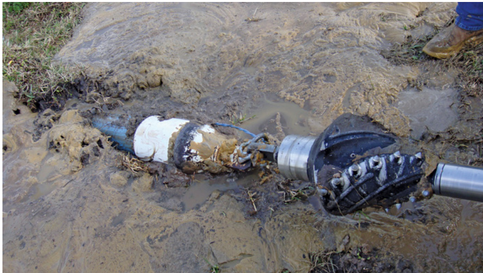
(Reprinted from "Tracer Wire System Importance for HDD" (2013) by Lee Dester with permission of Copperhead Industries, LLC)
