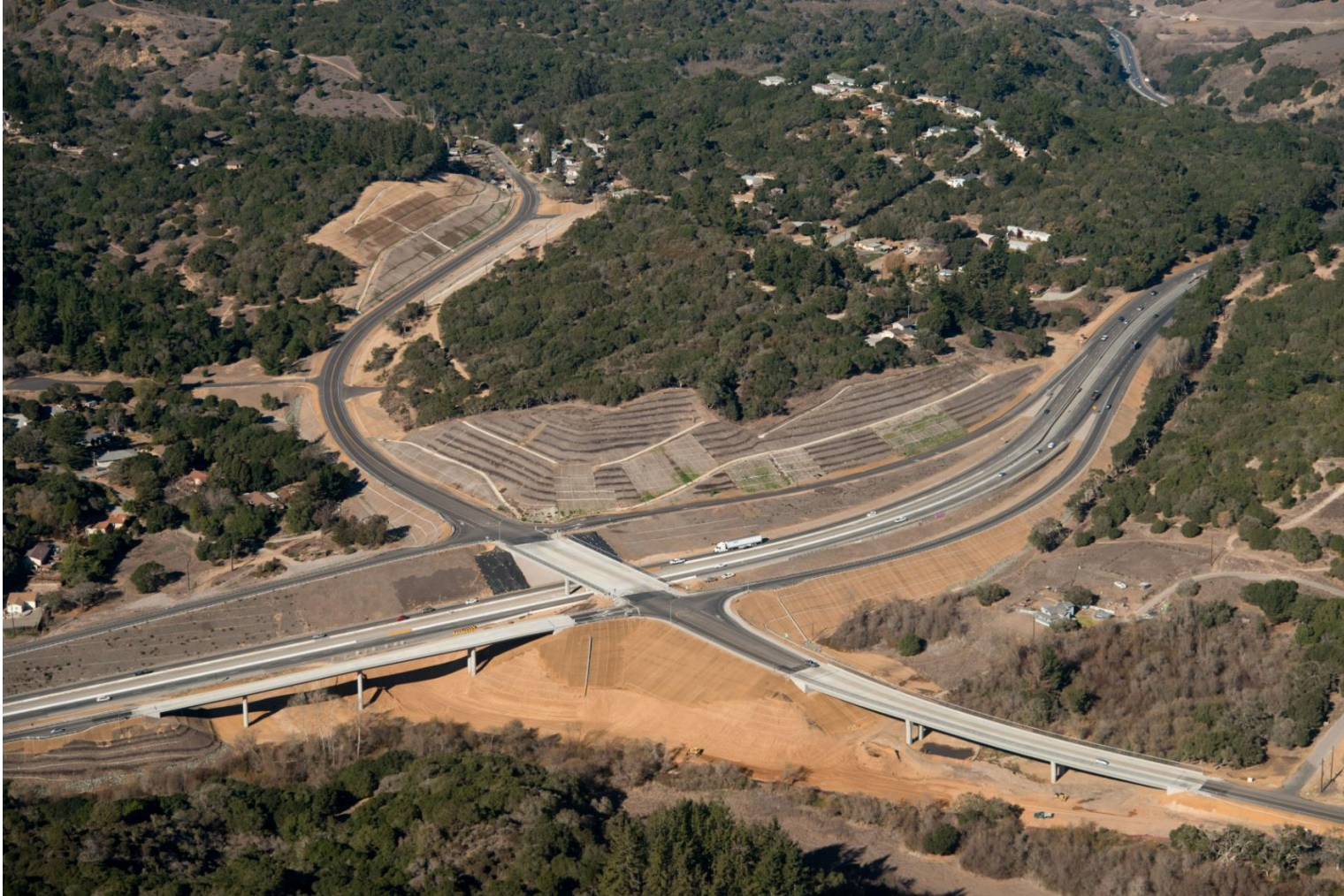
Hwy 101 Prunedale Improvement Project 45,000 cubic yards of compost used covering over 108 acres.
