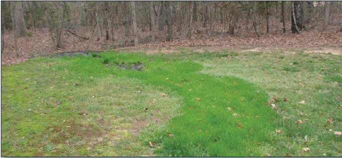
Figure 2. Surfacing of effluent from a failing septic system (repaired in 2009) is visible at the ground surface.
