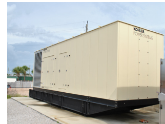
Power Supply and Electrical Components
