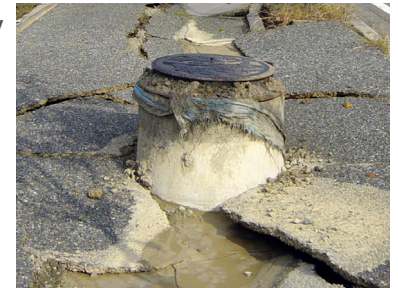
Manhole floats from liquefaction
