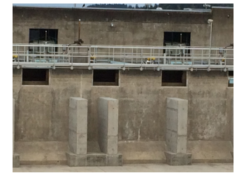
Basins, Reservoirs and Impoundments
