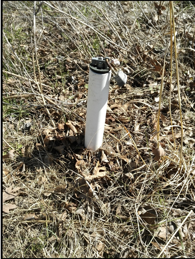
Picture 3: Monitoring Well W1
