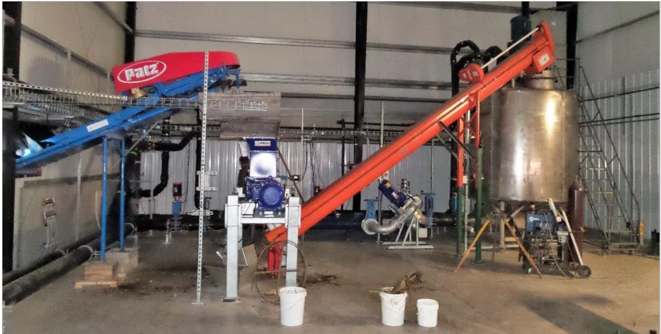
A Patz gutter cleaner conveys solid food waste into a grinder which then meters the waste into a stainless-steel vat where it is mixed with liquid manure and other liquid substrates. After mixing, the material is pumped into the digester. Photo Credit: EnviTec Biogas
