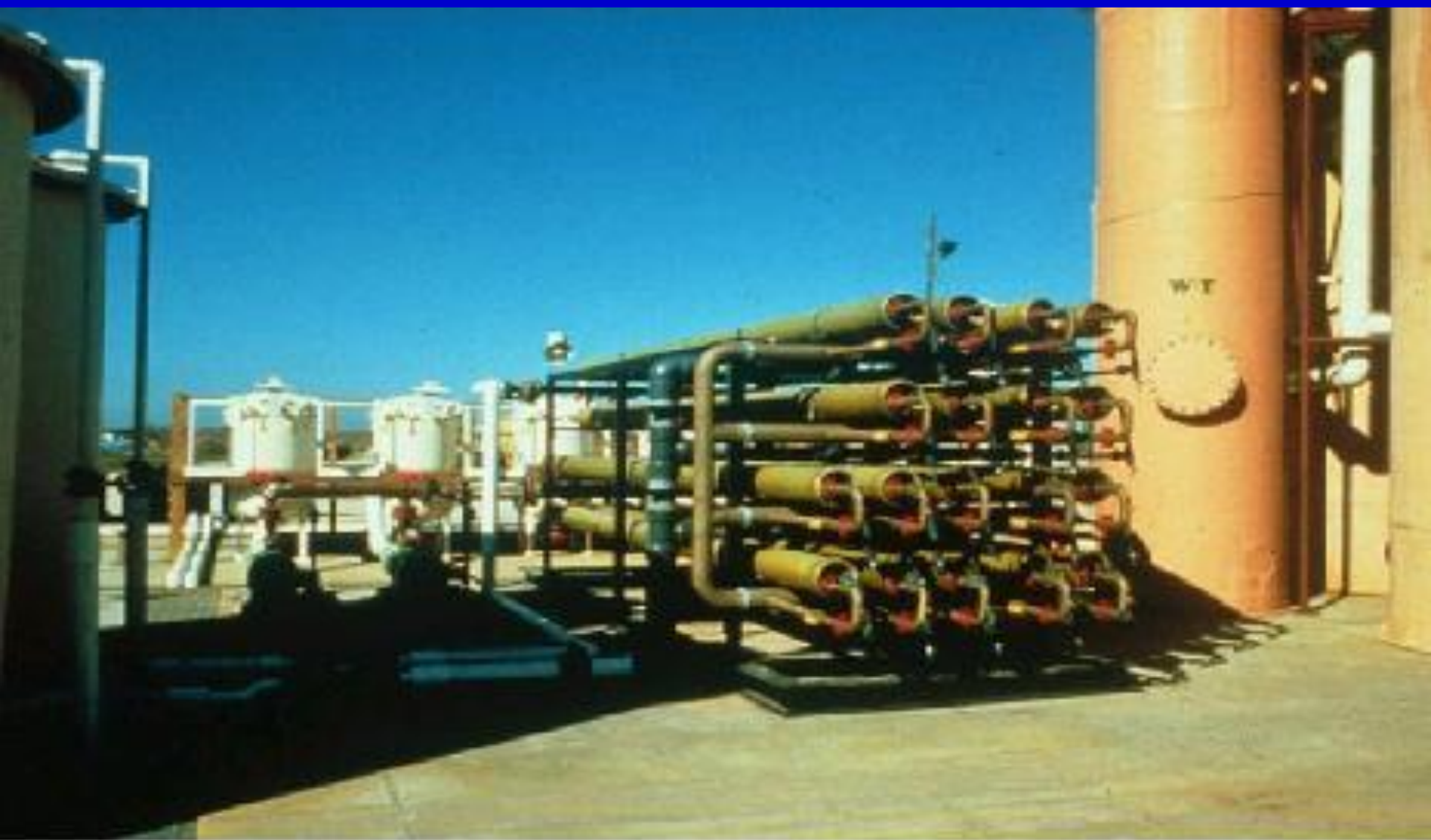
Reverse Osmosis Equipment
