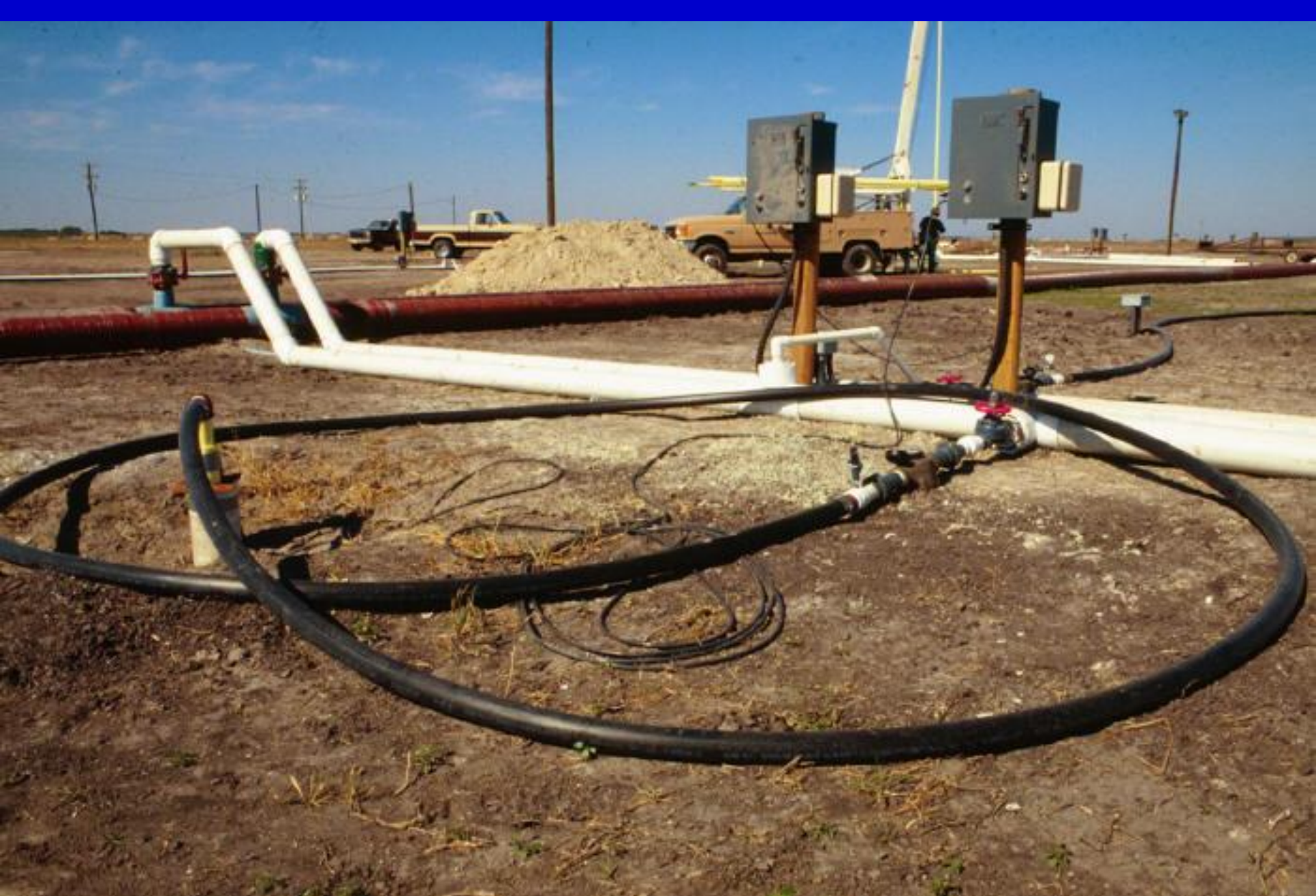
Flow Lines and Meters
