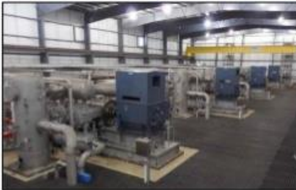
Four Compressor Train
