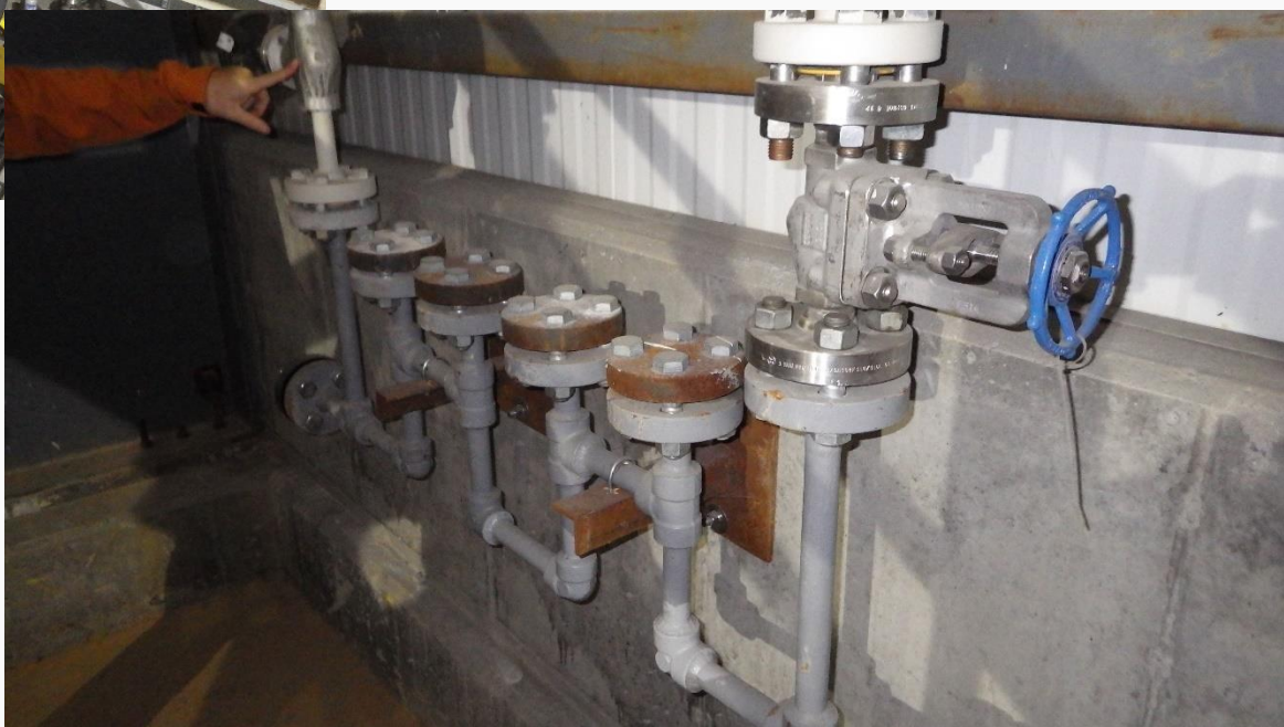
Corrosion Monitor Coupon Loop
