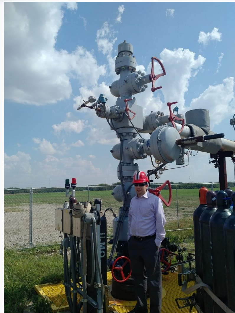
CCS #2 Finished Wellhead Injecting
