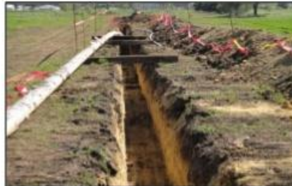
8" High Pressure transmission Line
