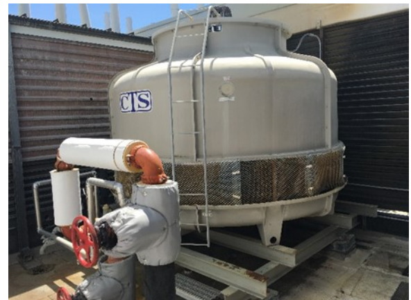
Figure 5. Two 150-ton cooling towers are operated in sequence to provide building cooling in the main building.
