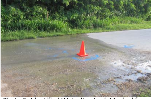
Photo 5: Identified Waterline Leak Marked for Repair (photo courtesy of David Hidalgo, CUC)
