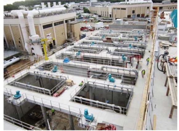
Photo 3: Blue Plains Filtrate Treatment Facility (photo courtesy of PC Construction Company)
