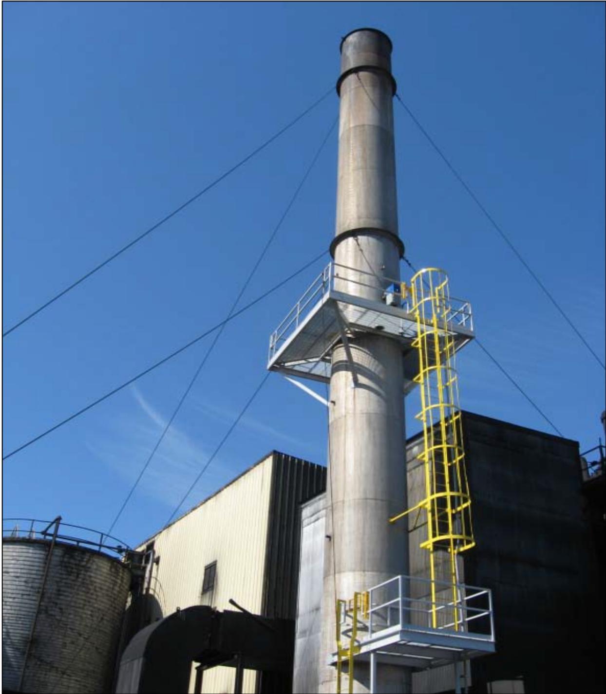
Figure 1-2. Example of a Ducted Stationary Source Stack
