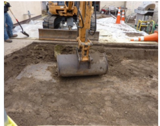
Colorado Smelter cleanup crews excavate contaminated soil from a residential property in Pueblo, Colorado
