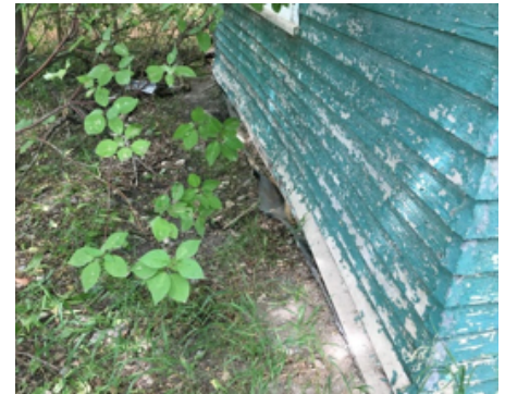
Brownfields Cleanup, Spirit Lake Reservation. Photo of an abandoned building contaminated with asbestos, lead-based paint, and lead in the soil.
