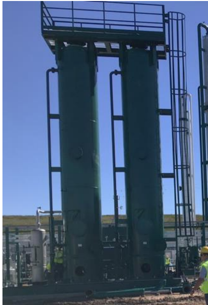
Sulfur removal vessels at a Solvent plant
