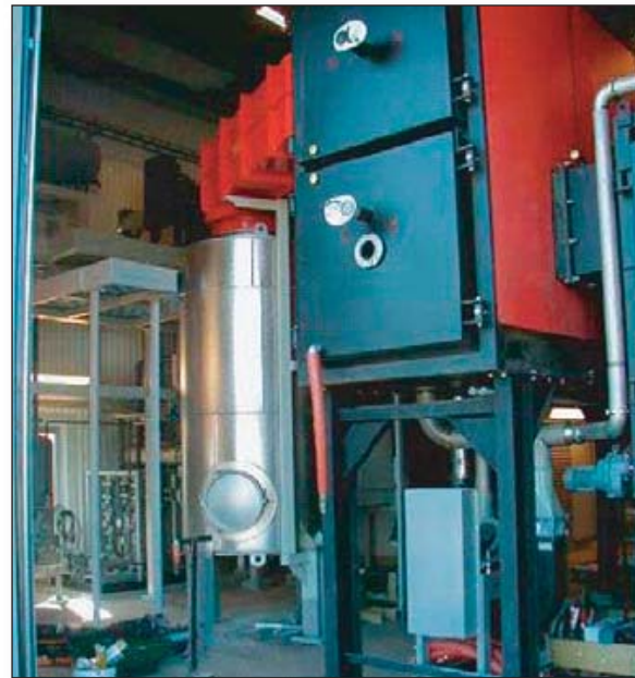
BioCon® ERS Unit (Photo courtesy of Kruger USA).
