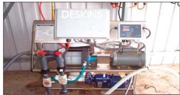
Polymer Preparation Unit
