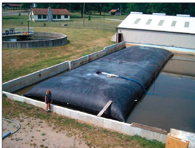
Geotube® Container at Cambridge WWTP after being filled with 250,000 gallons of biosolids. (Mastin and Lebster, 2006).
