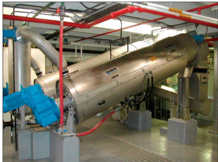
Installed incline screw press at Old Town Water Pollution Control Facility. (Atherton et al., 2005)
