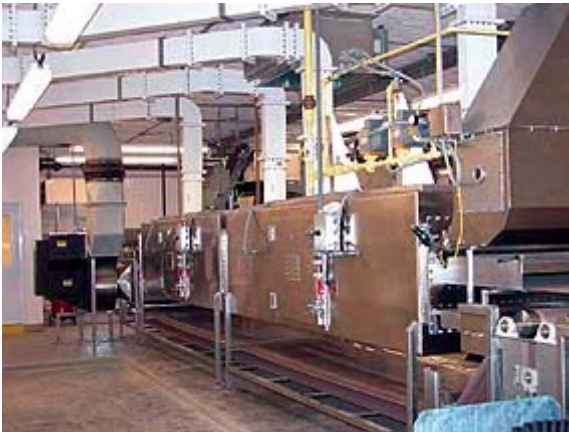
Burch BioWave ® dryer installed
