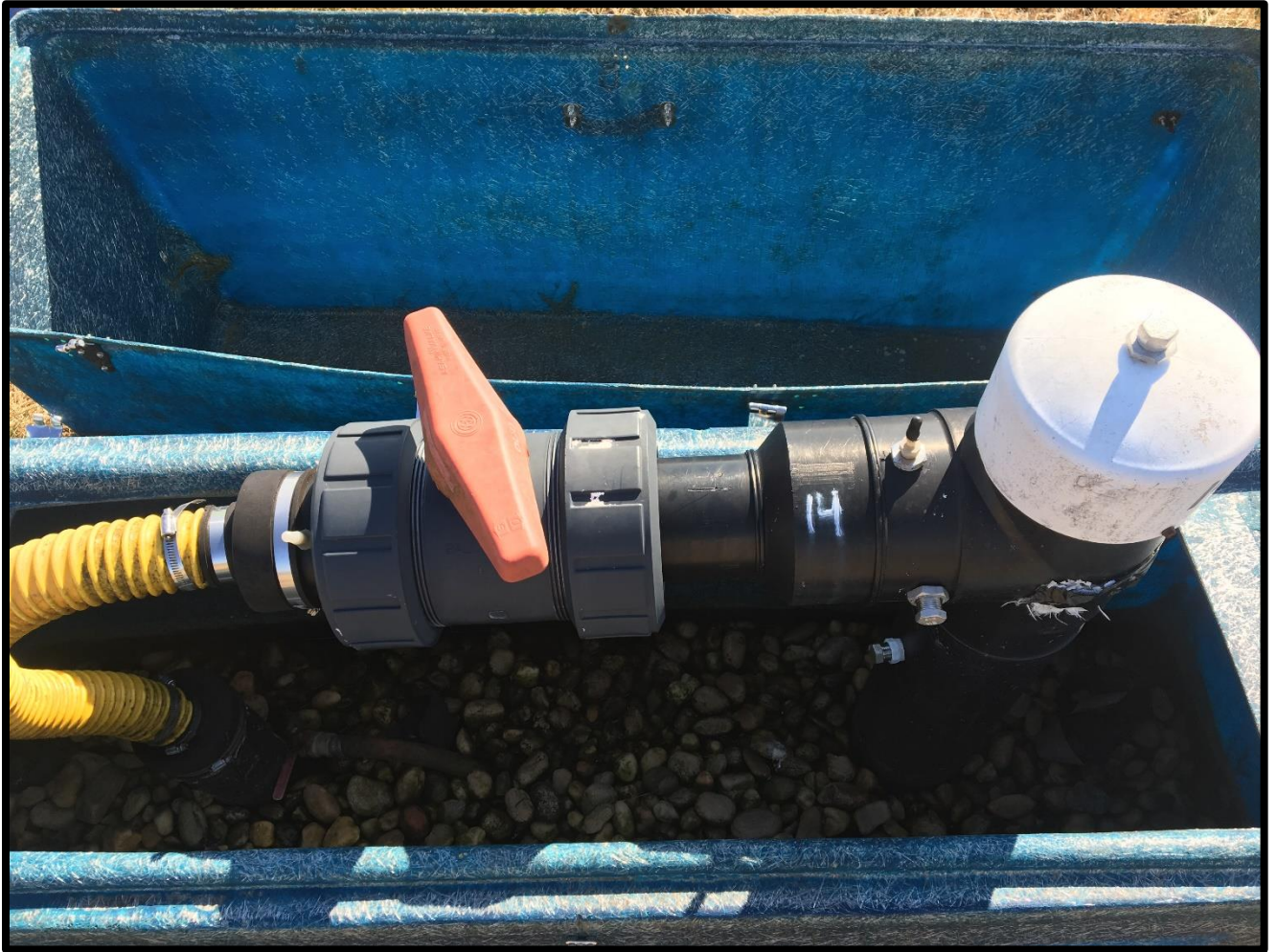
Picture 6: Gas Extraction System well #14
