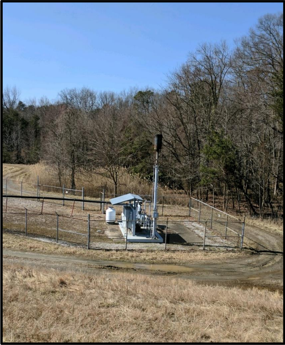
Picture 5: Methane Gas Extraction System candlestick flare
