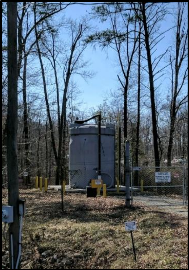
Picture 8: Leachate storage tank
