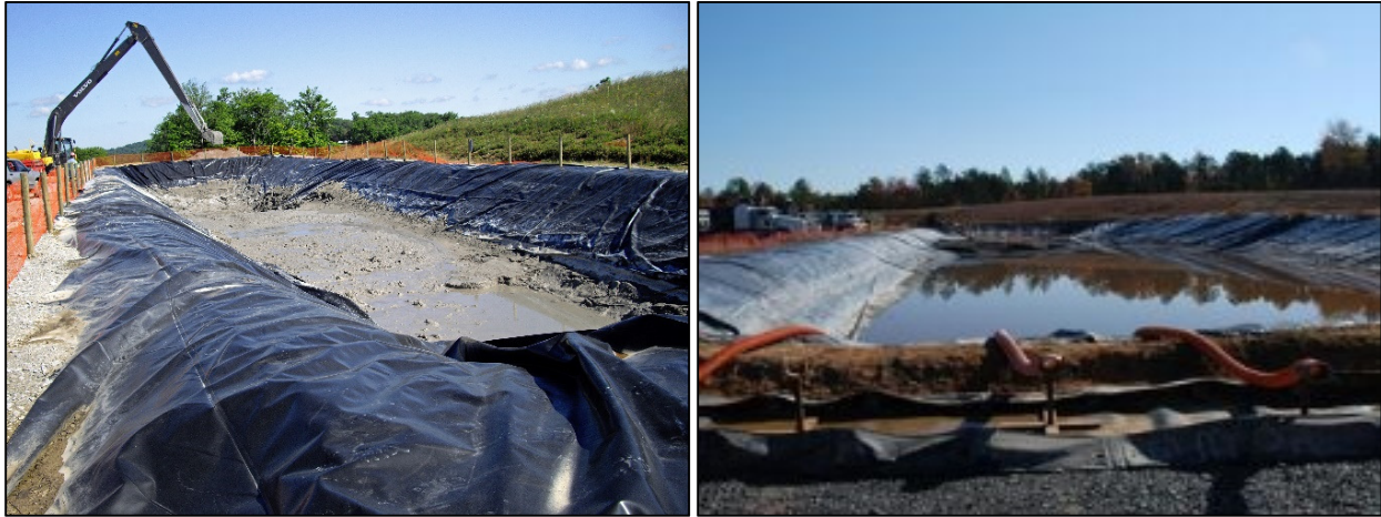
Figure 4-1: Pits with Visible Liners.
