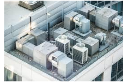
HVAC: Improved Building Filtration System
