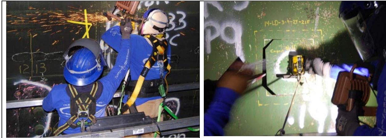
Figure 3-1 Coupon Removal Tank 14
