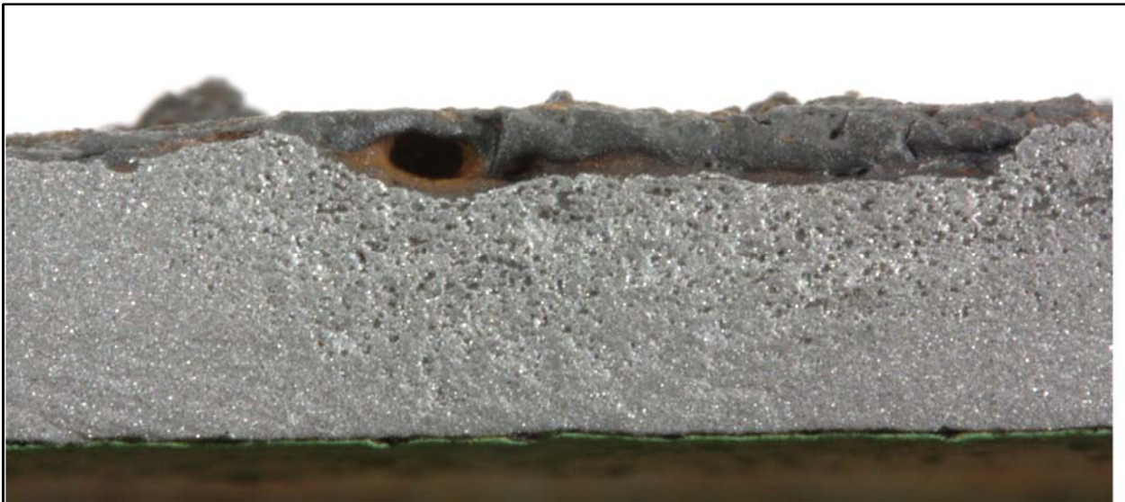
Figure A-4. Detail of the sandblasted edge on 3/20/19 in the same location as shown in the picture below. The sandblasting revealed that the feature was not a corrosion pit, as shiny metal was revealed when the red-colored staining was removed. There was an unusual appearance to the edge in this location, as though the sectioned edge had been superficially altered by heat associated with sectioning or some other post-sectioning reaction (atmospheric corrosion or corrosive media attack). That alteration gave the appearance of a deep corrosion pit.
