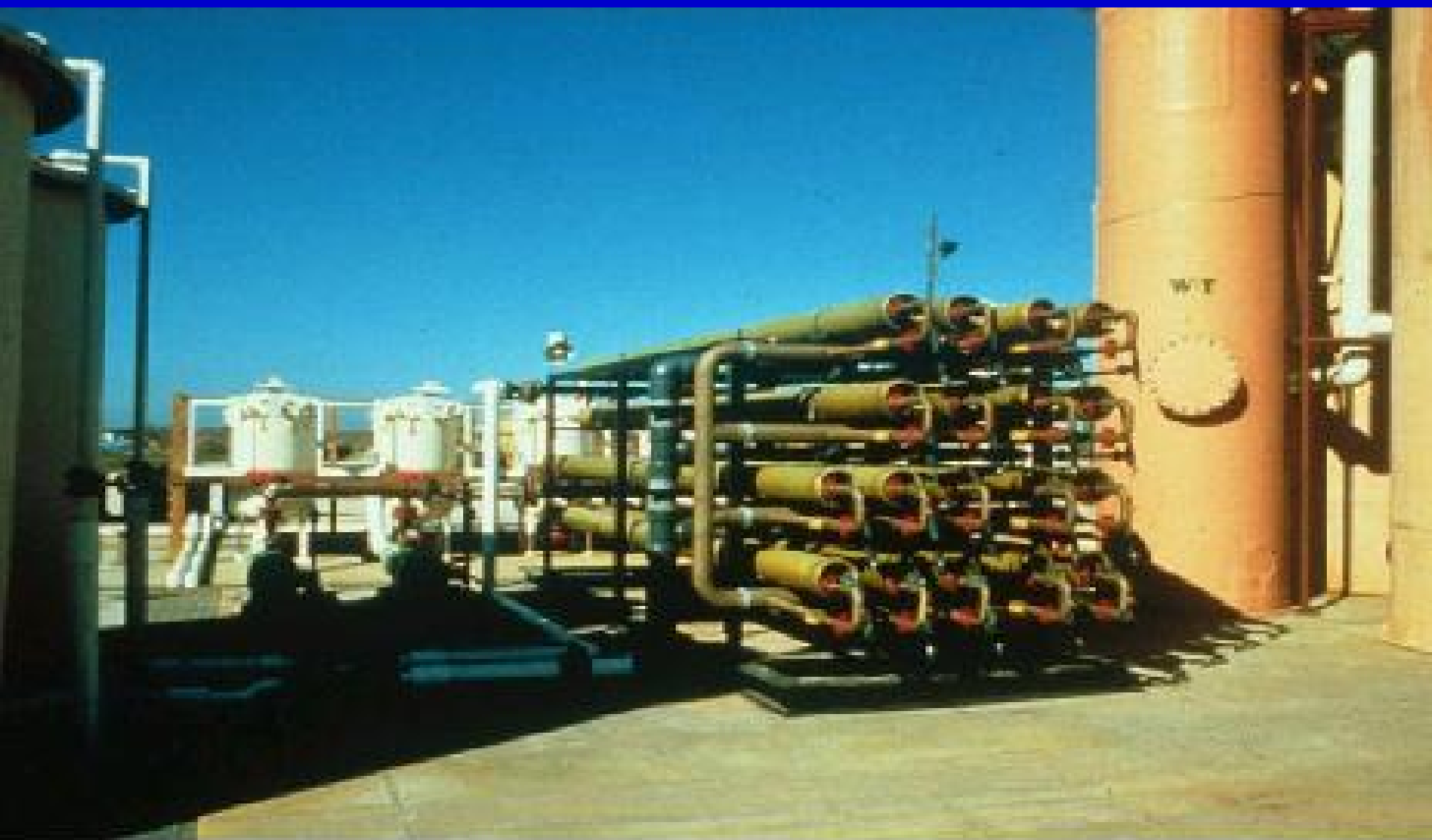
Reverse Osmosis Equipment
