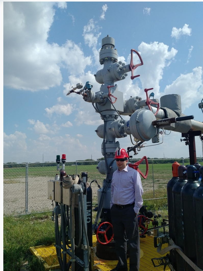
CCS #2 Finished Wellhead Injecting
