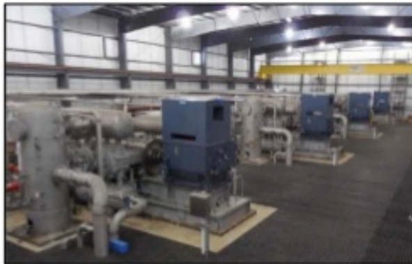
Four Compressor Train
