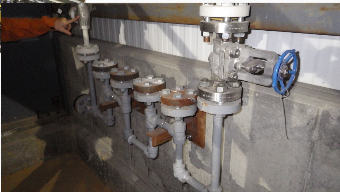
Corrosion Monitor Coupon Loop
