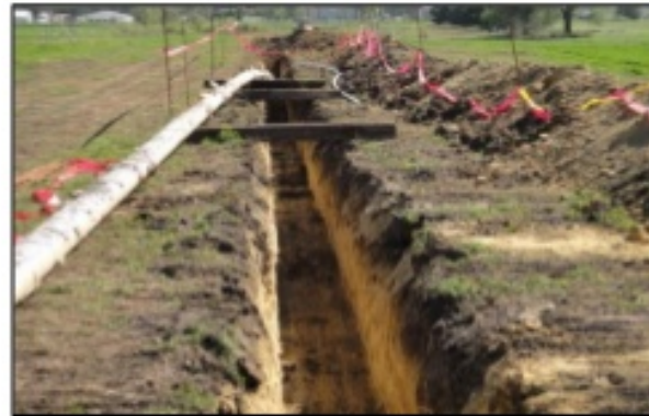
8" High Pressure transmission Line
