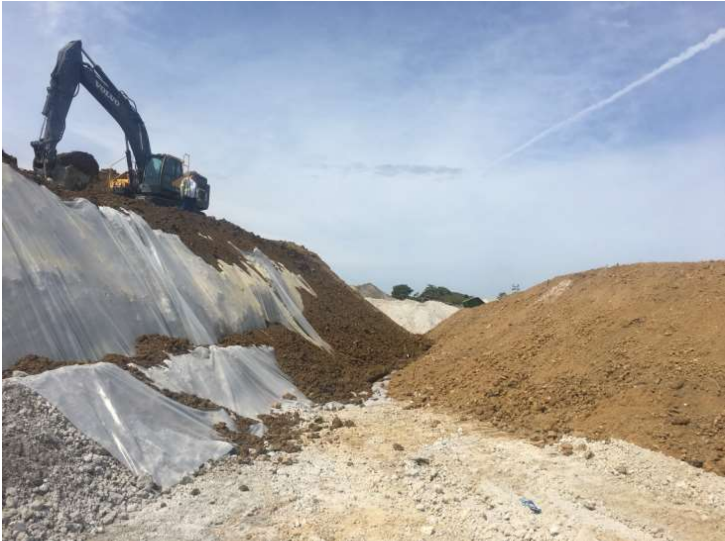
Capping slag excavation face and contaminated slag pile with plastic and clean fill
