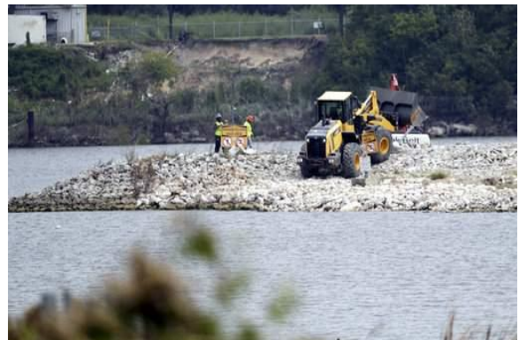
Repair of the San Jacinto Waste Pits cap armor following Hurricane Harvey.
