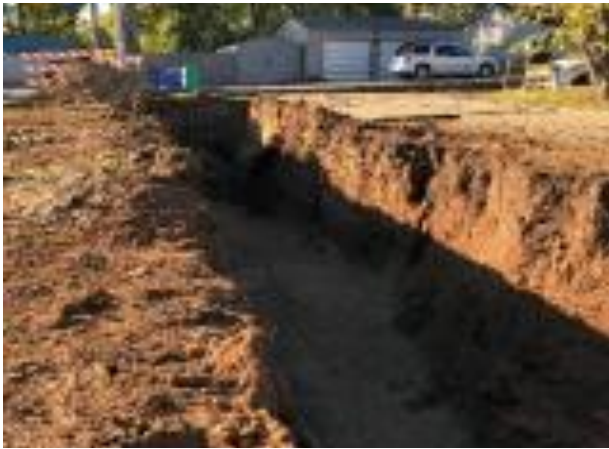
Trench where 245 feet of the old sewer line and 340 tons of contaminated soil were dug out on the former Amphenol site north of Hamilton Avenue in October 2019.
