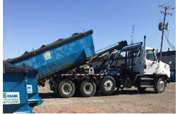
Nearly 7,000 tons of impacted soil were dug up and sent to a landfill in the blue containers shown here.
