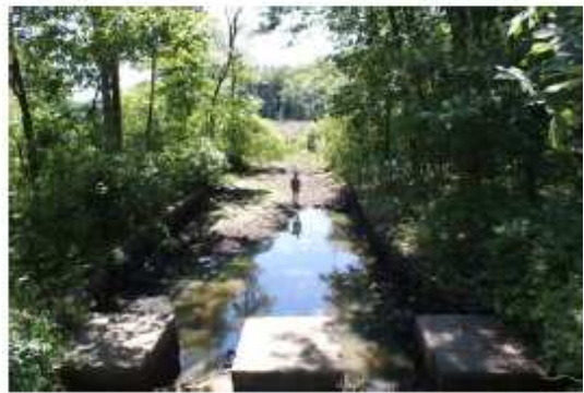
Martins Brook dry streambed at Rt. 62 crossing and weir. Taken 8/3/2016, Wilmington, MA. Lat. 42.579646, Long. - 71.138928
