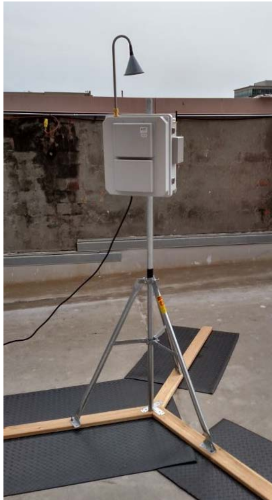
Figure 2. MOB box installed at the 6 th & Jackson site.
