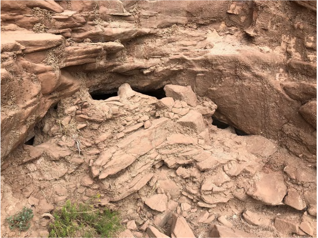
Photograph 4. Reclamation compromised due to unnatural drainage at a portal above Haul Shaft.
