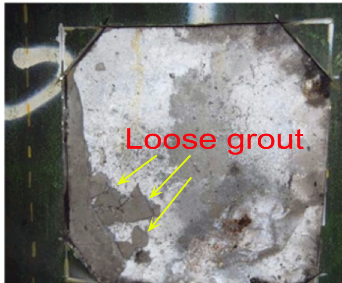
Figure 10: Loose grout behind coupon plate P6. From DT Results Report [1].
