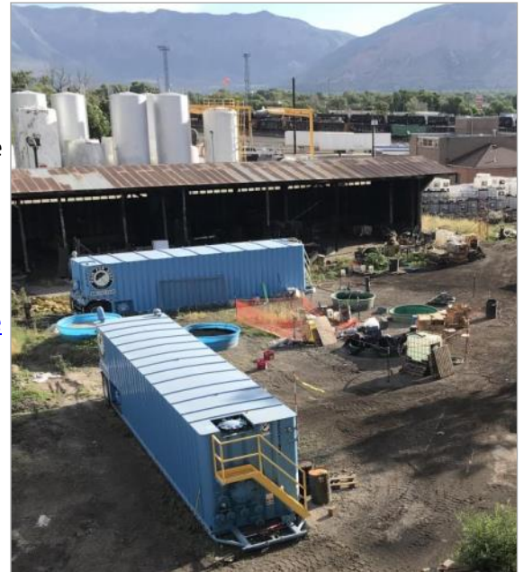
On-site wastewater treatment
