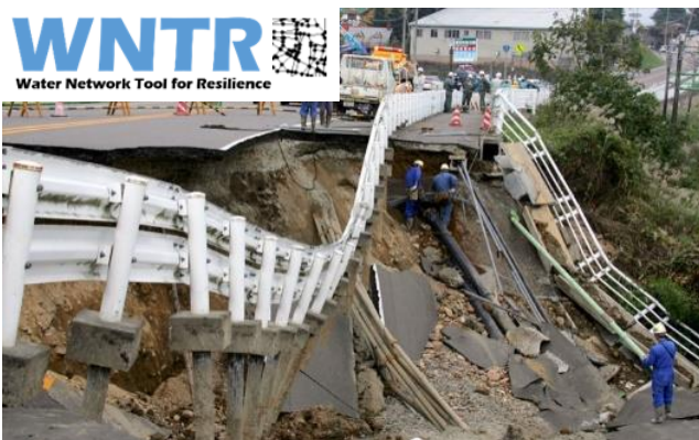
Figure 1: Damage following earthquake, including broken pipes.
