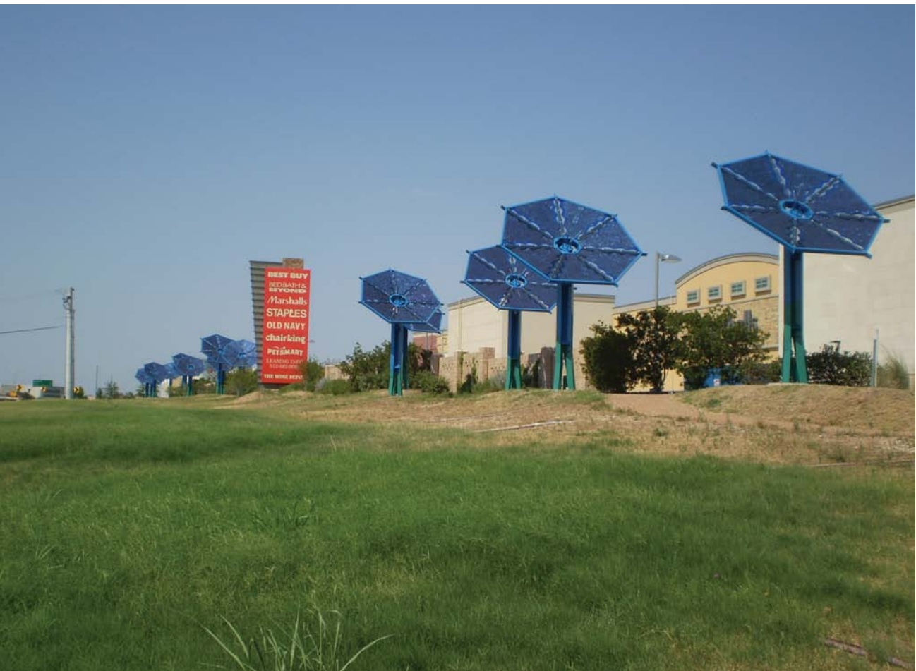
Located along Interstate 35, near Austin, Texas, is a PV installation of 15 Mueller PV sunflowers. (Vipin Gupta/PIX17928)
