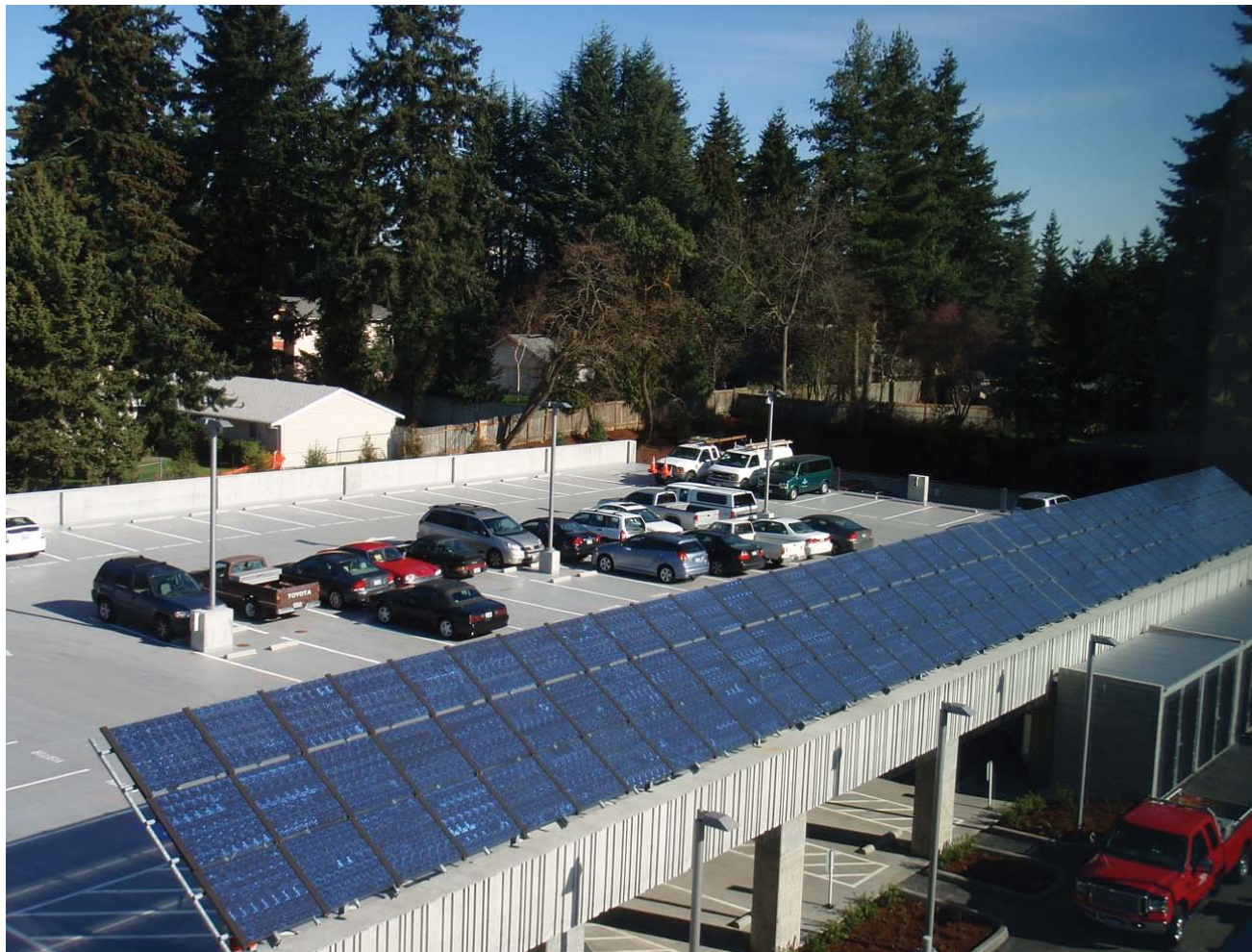
The City of Shoreline, Washington, installed a 20.2 kW solar electric system on top of the City Hall parking garage. The system uses Washington-made solar modules from Marysville-based Silicon Energy. (City of Seattle/PIX18074)
