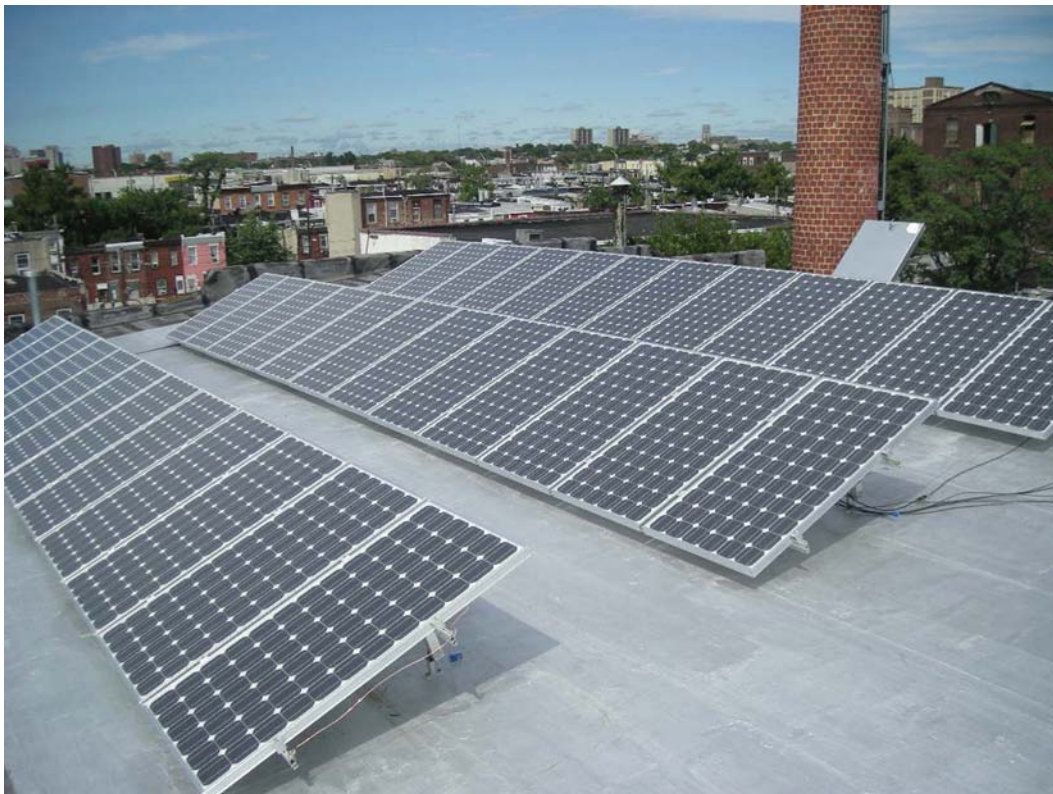
Mercury Solar Systems installed this 6 kW installation in the Lower Kensington neighborhood of Philadelphia. (Mercury Solar Systems/PIX18065)
