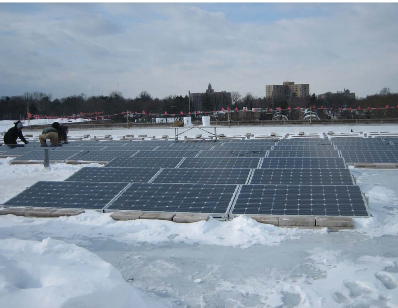
Nearly 2,000 solar panels installed at the Veterans' Affairs Regional office and Insurance Center in Philadelphia produce over half a million kilowatt-hours of solar electricity annually. (The U.S. General Services Administration/PIX18066)
