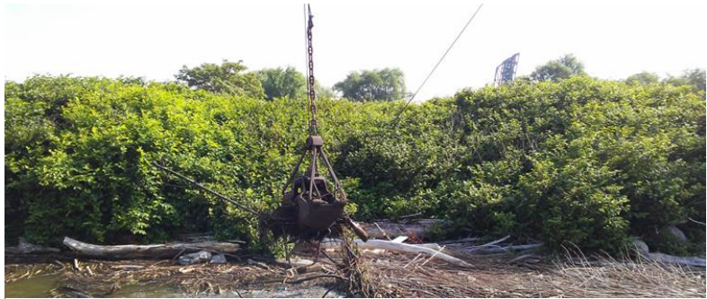
Figure 15. Three barges of large woody debris were removed from the “Blue Tower Turning Basin” site. The debris was removed from this site before in-water habitat was planted. A rootwad chain and floating boom system was then installed to deflect additional accumulation of debris.
