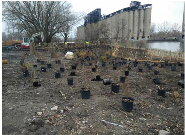
Figure 14. Trees ready for installation following invasive species treatment at the Toe of Katherine Street. Turtle nesting habitat was also created at this site.
