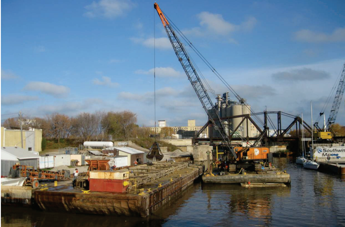
11. After dredging, Ryba placed sand cover using a specially designed sand spreader for thinner areas (6 to 12 inches) and a conventional clamshell bucket for thicker areas (up to 3 feet). This photo shows the conventional clamshell bucket in use.
