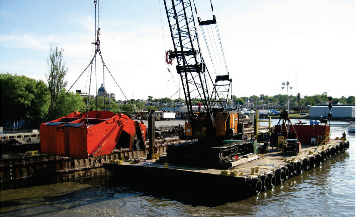
5. A 6-cubic-yard Cable Arm Environmental Level-Cut clamshell bucket was used for removal of sediments.
