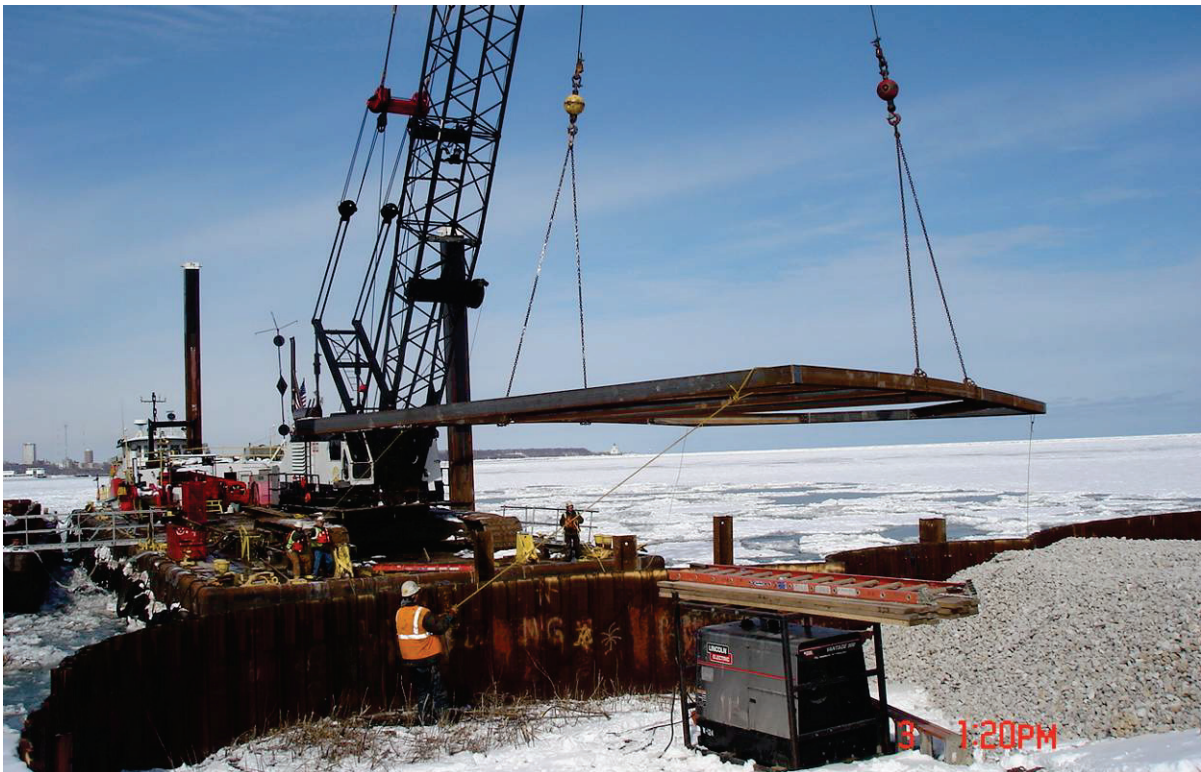
2. The Edward E. Gillen Company (Gillen) constructed the offloading platform at the Milwaukee Harbor CDF. In this photo, the pre-constructed waler system for the offloading platform is being lowered into place as the Gillen employees use taglines to control the load and maintain a separation distance from the overhead hazard.
