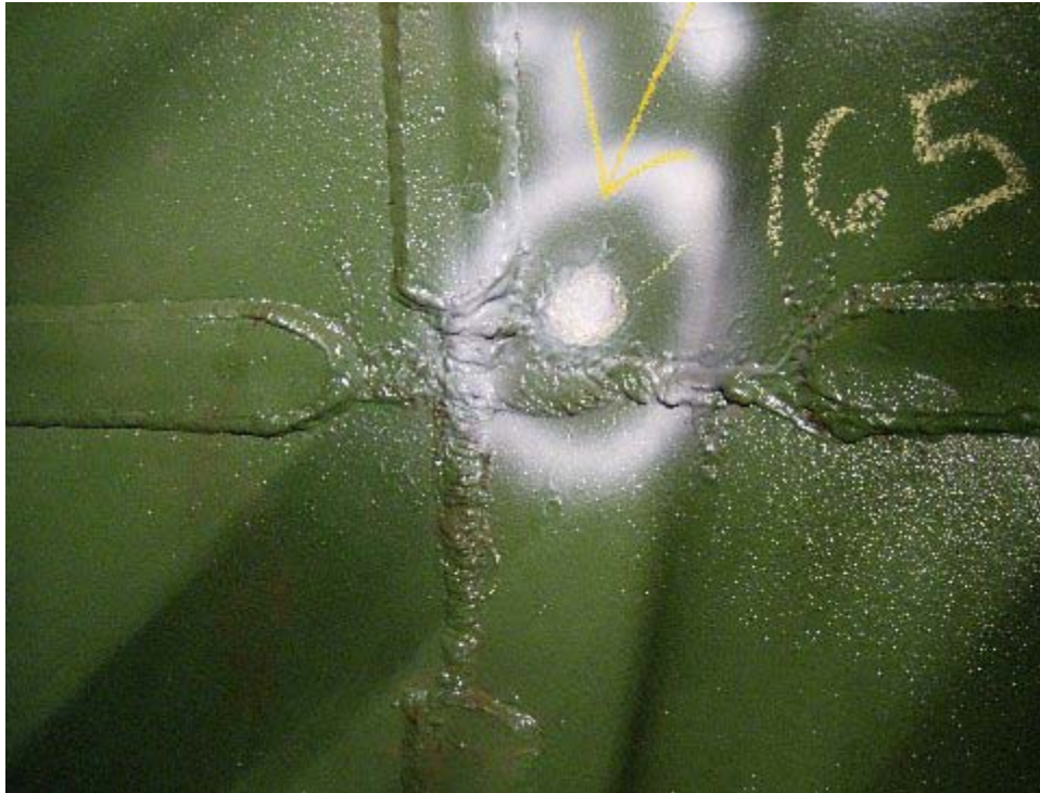
Flaw 304 Loss of Wall measured .165"
