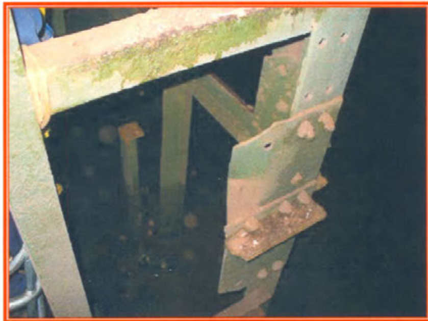
Photo #8: Missing diagonal
