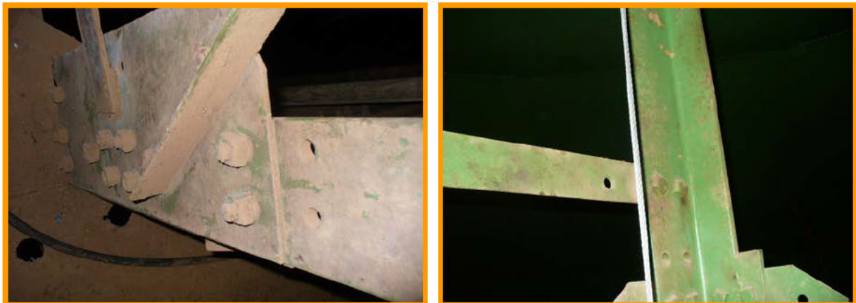
Image 1: Showing Tank #20 Tower frame and boom missing members and bolts
