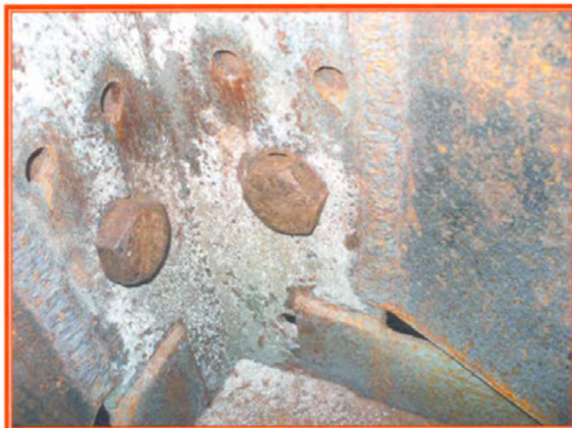
Photo #2: Visible slippage of the bolt connection
