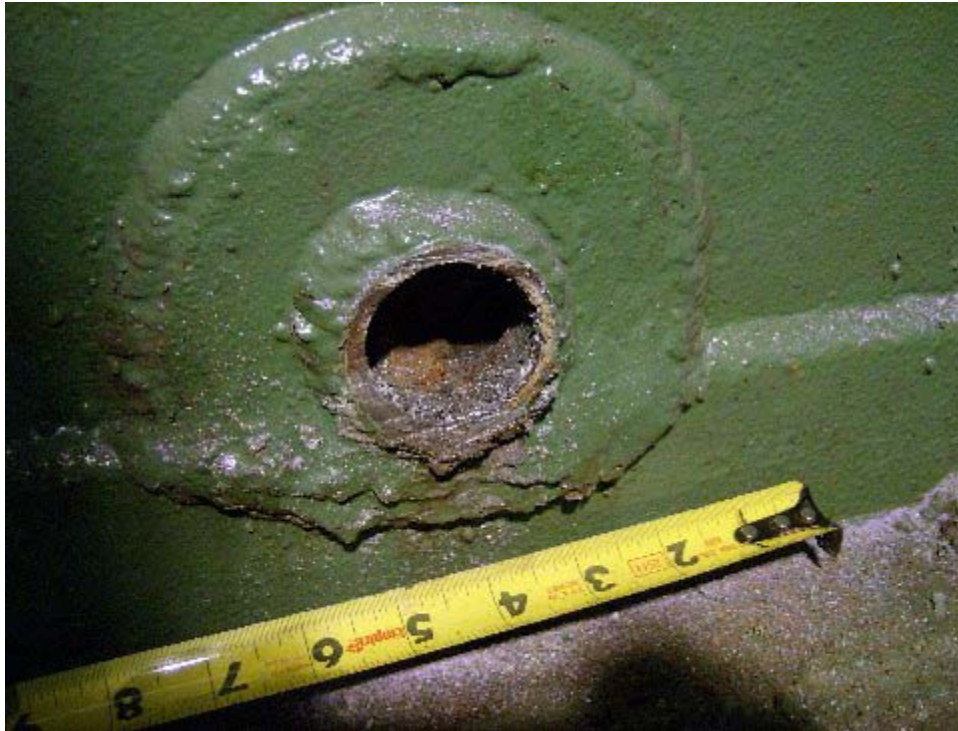
One of approximately Six Hundred piping penetrations that were removed requiring repair
