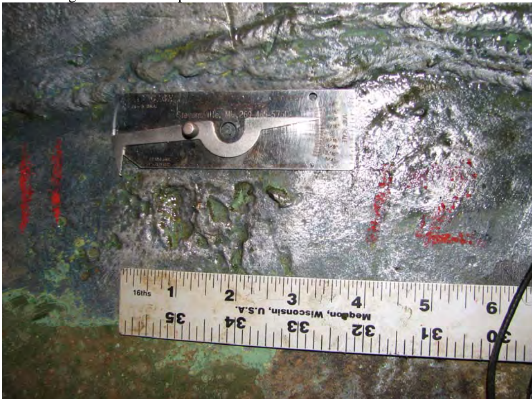
Flaw # 83, topside pitting on plate 4 of the floor, 0.336" remaining, near plates 11 and 12 of course 1
