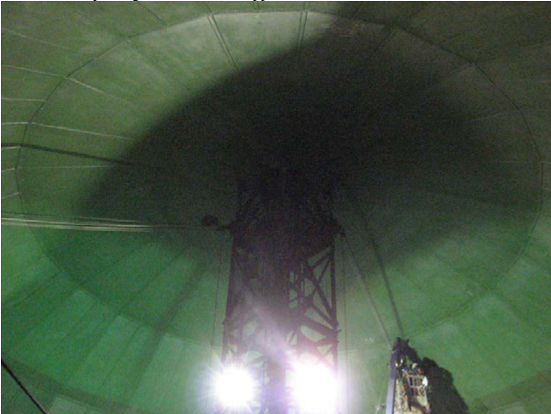
A view of the very top of tank # 2 showing courses D, E, and F with a TesTex crew
