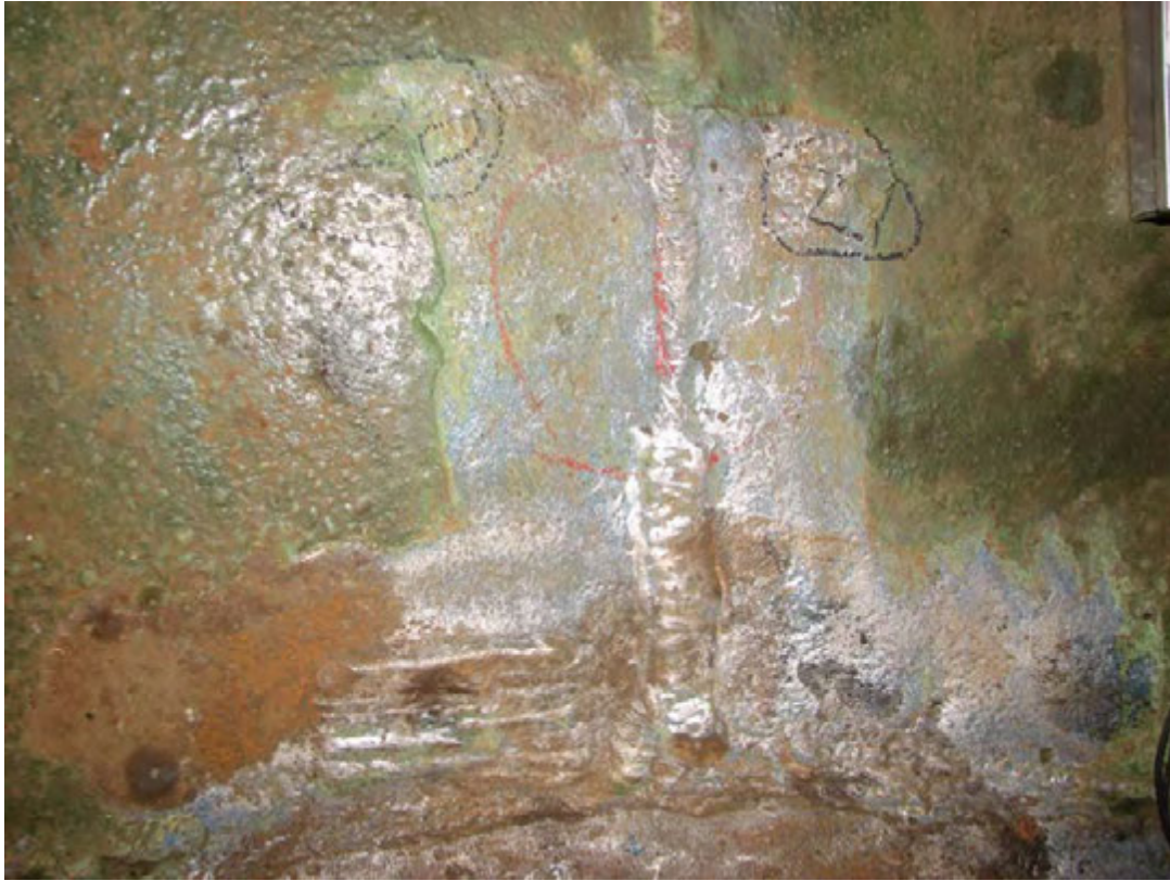
Intersecting welds between plates 20 and 21 of course 1 and the floor.
