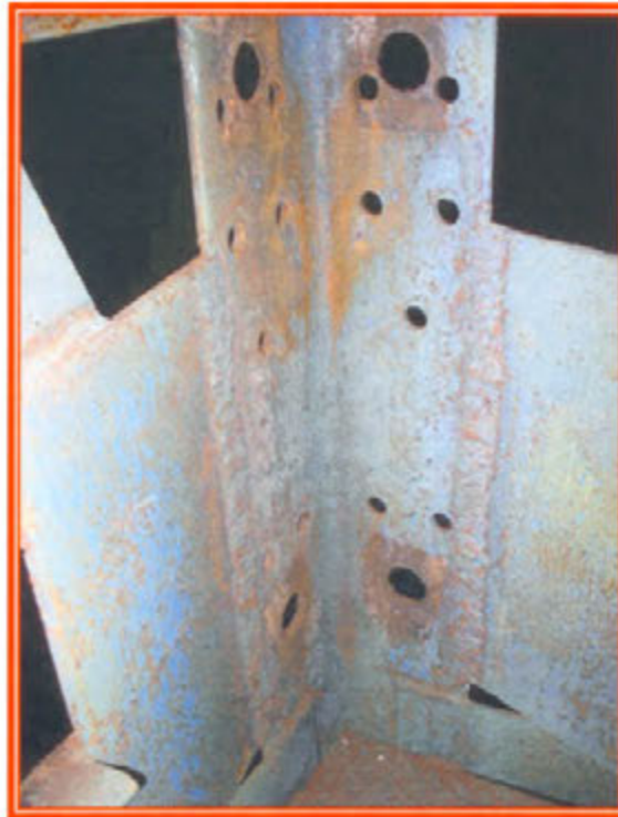
Photo #3: Big holes on the framing members
