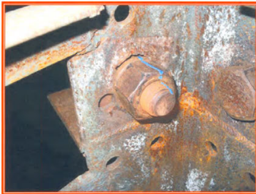
Photo #1: Visible slippage of the bolt connection
