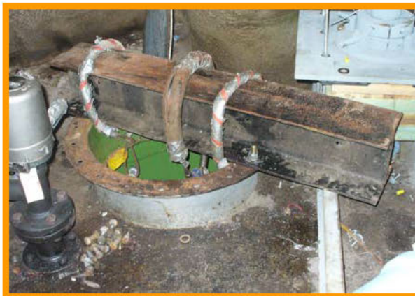
Image #3: Showing Tank #20 Spider hoist assembly top anchoring
