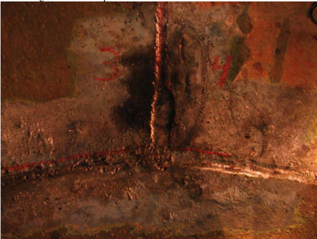
Intersecting welds between plates 3 and 4 of course 1 and the floor.
