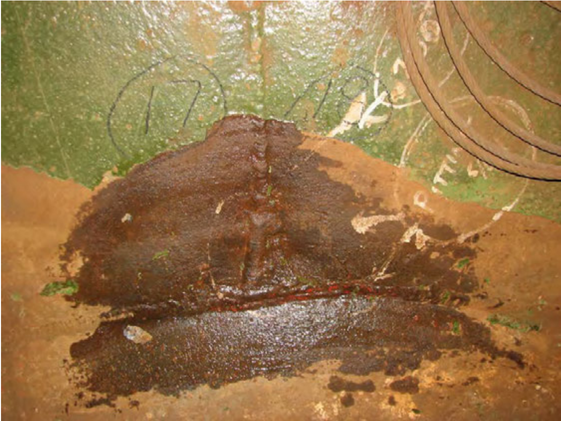
Intersecting welds between plates 17 and 18 of course 1 and the floor.
