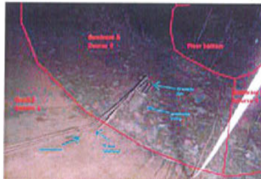
Paint / Coating – Chips and pieces along the bottom after pressure washing.
