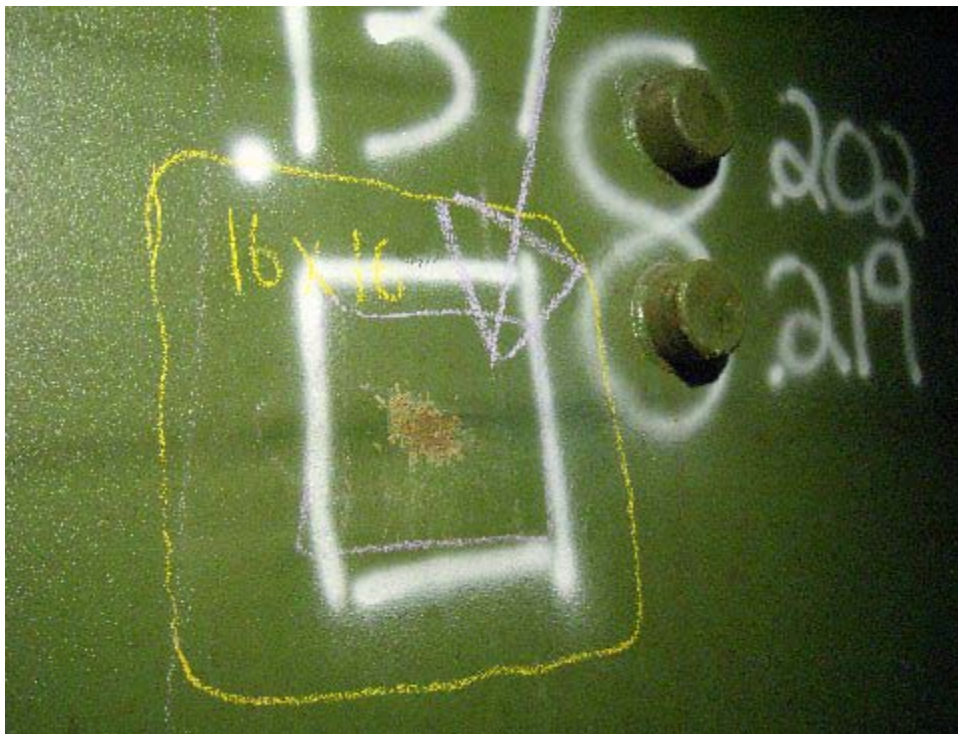
Location of Flaw 334 Underside corrosion at .137" requiring a 16" X 16" Lap Welded Patch
