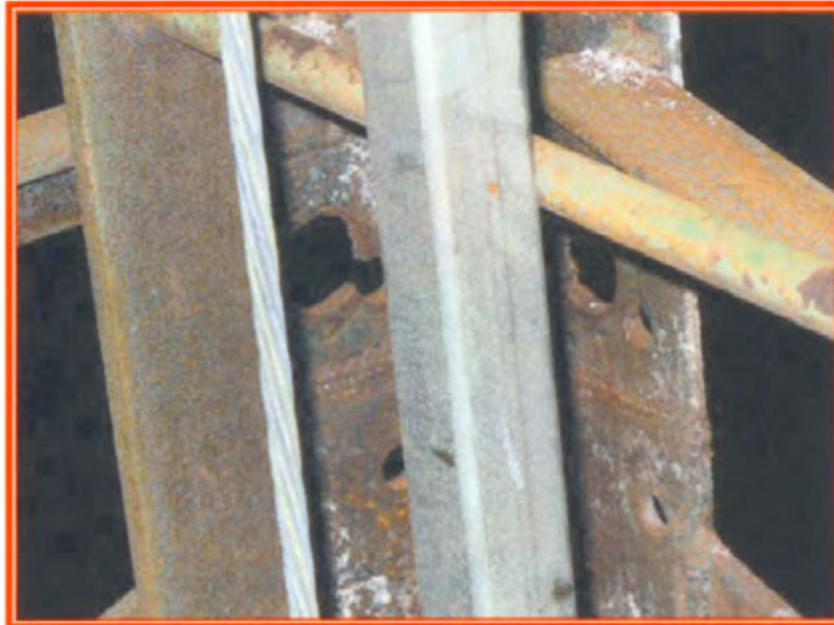
Photo #4: Big holes on the framing members
