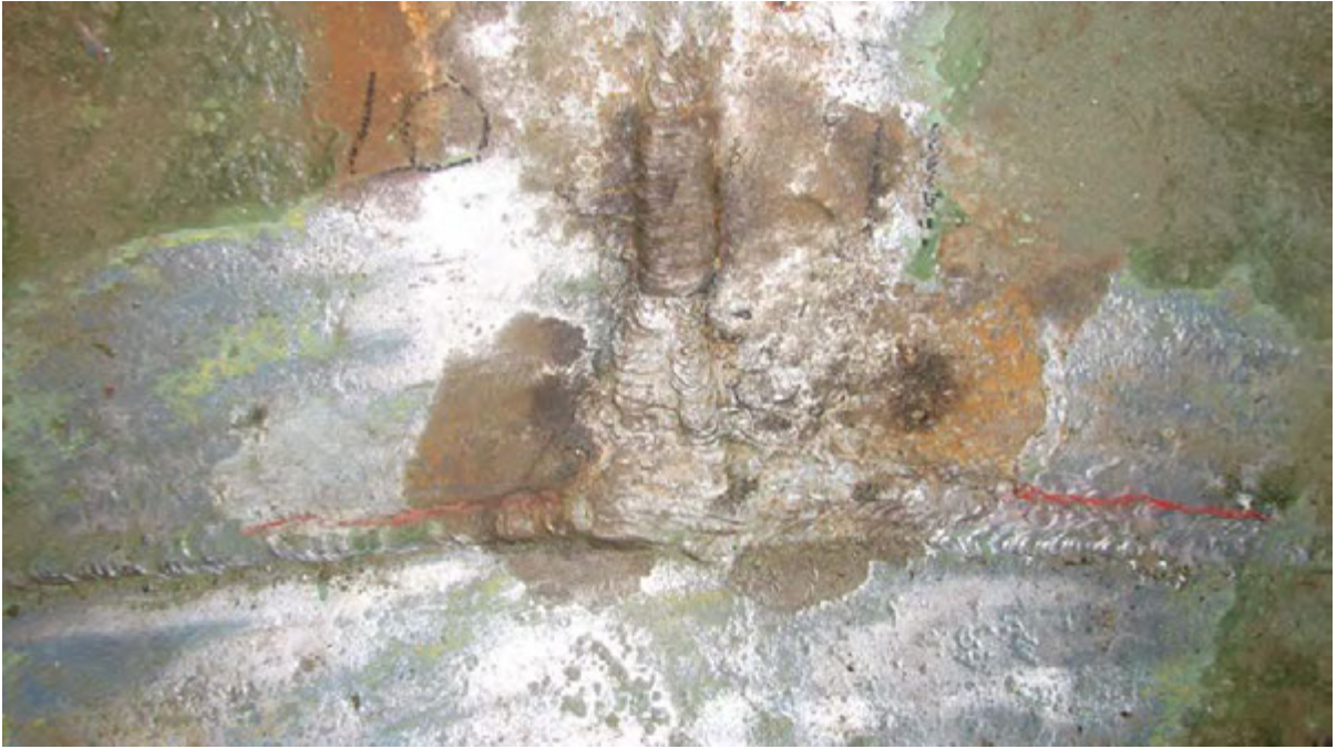
Intersecting welds between plates 10 and 11 of course 1 and the floor.
