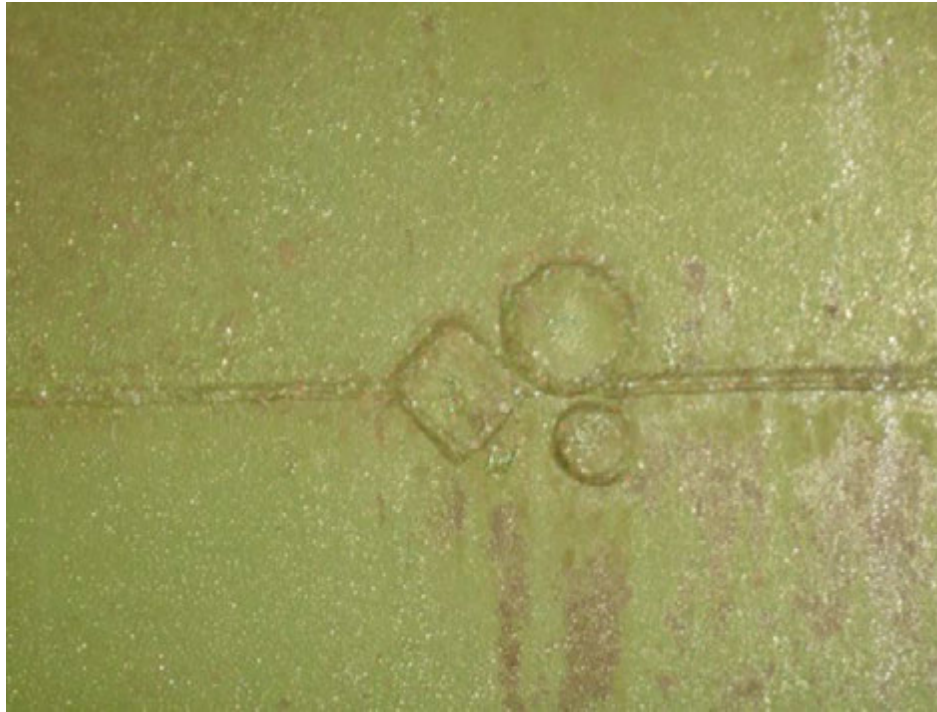
Existing Lap Patches in the Barrel section of tank 20 Note: Coating condition
