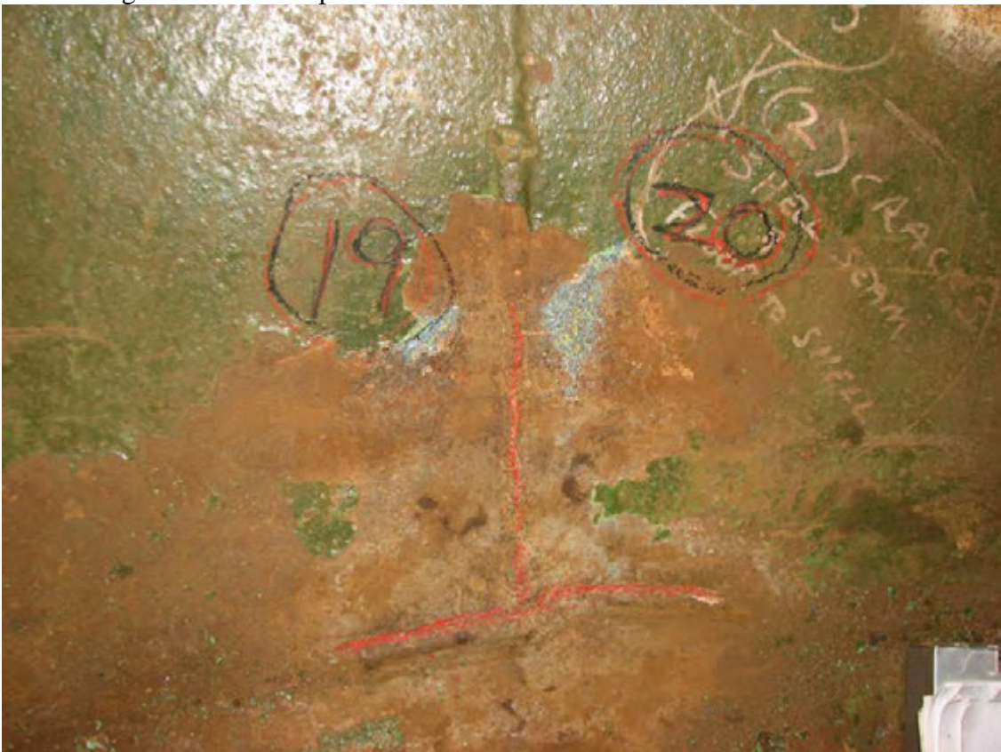
Intersecting welds between plates 19 and 20 of course 1 and the floor.
