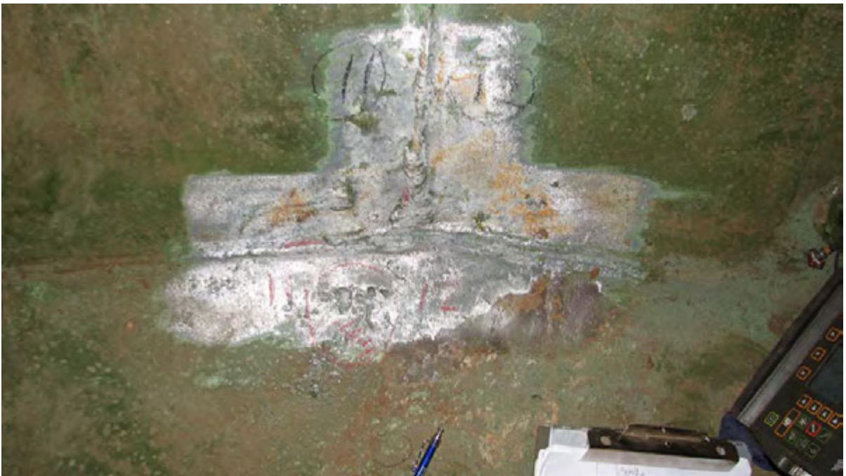
Intersecting welds between plates 11 and 12 of course 1 and the floor.
