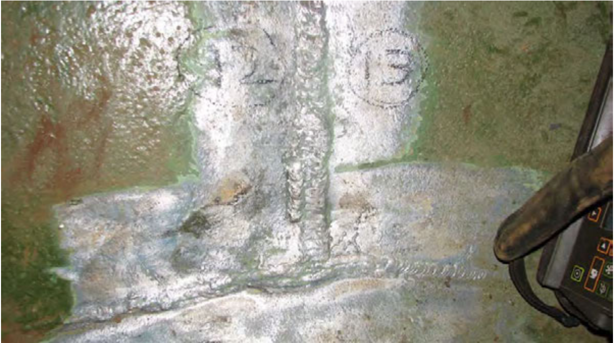
Intersecting welds between plates 12 and 13 of course 1 and the floor.
