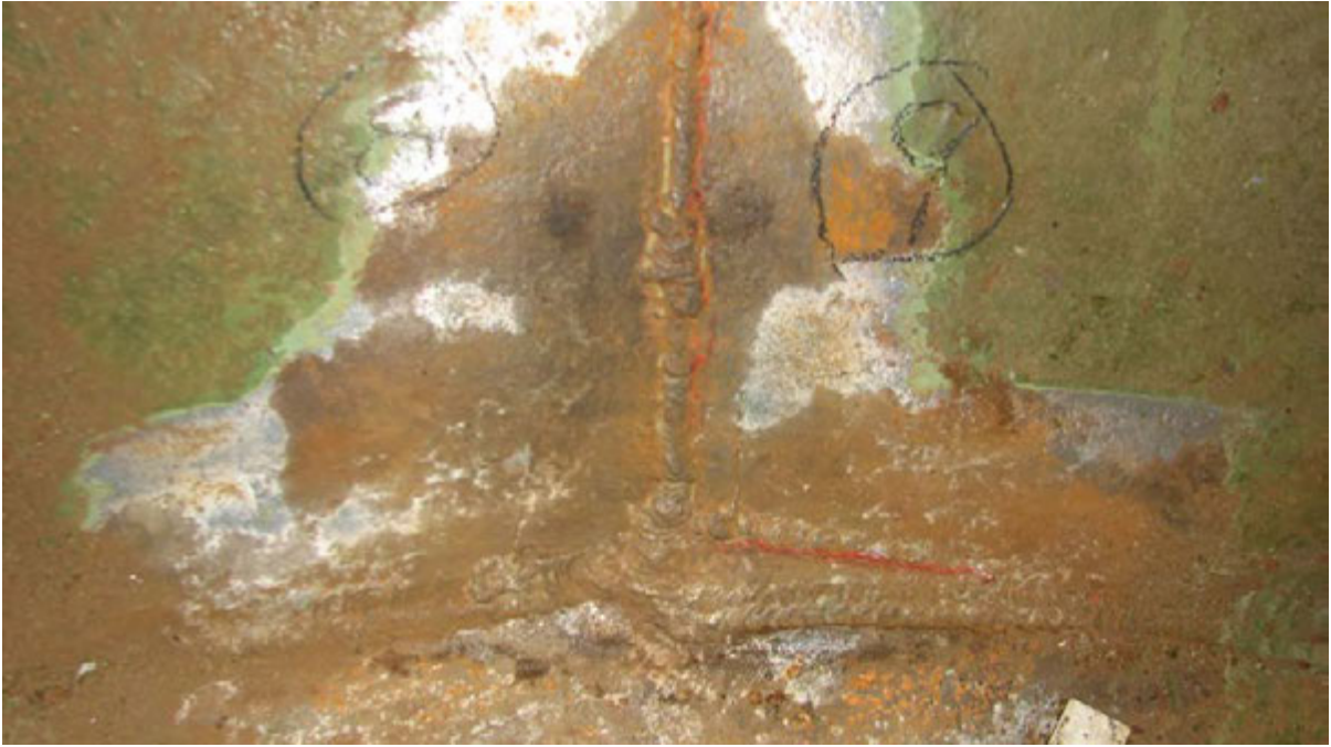
Intersecting welds between plates 8 and 9 of course 1 and the floor.
