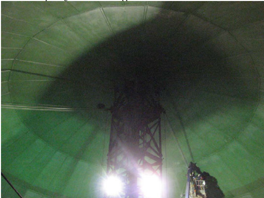
A view of the very top of tank # 2 showing courses D, E, and F with a TesTex crew
