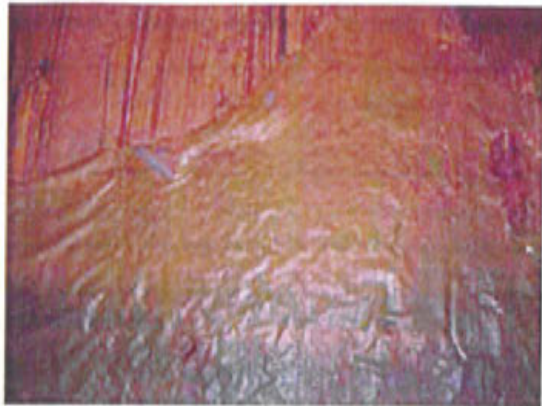
Paint / Coating – Disbonded & blistered
