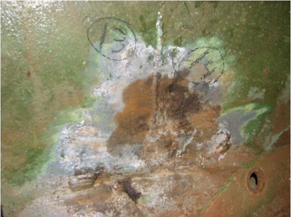
Intersecting welds between plates 13 and 14 of course 1 and the floor.
