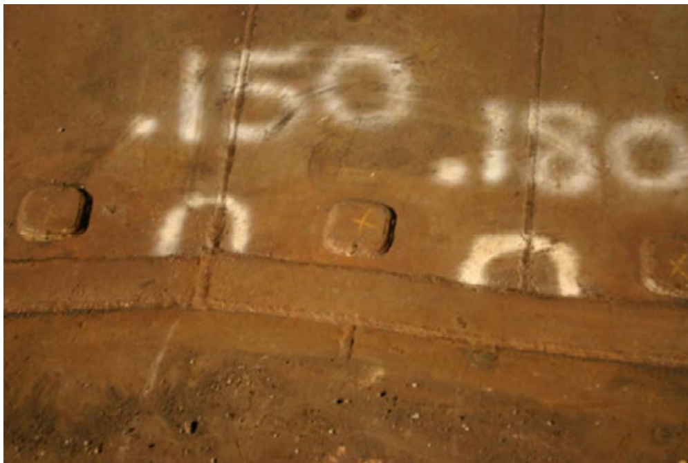
Photograph 12 – Lower dome and the bottom of the tank. Note the flaws marked at the intersection of the lower dome plates and bottom plates.
