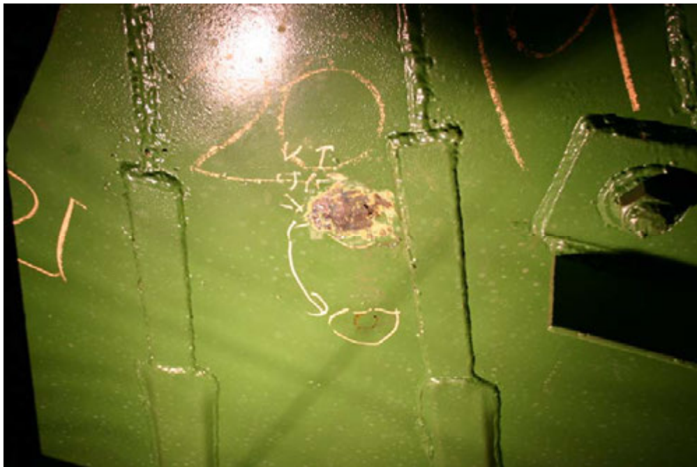
Photograph 8 – Holes at the top of course F of the upper dome.
