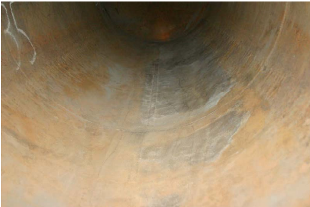
Photograph 10 – The same section of piping after the poorly adhering thick-film coating was removed. UT measurements indicate that the corrosion in this area of the pipe is not extensive and the coating appears unnecessary and somewhat ineffective when the surface preparation is not completed correctly.
