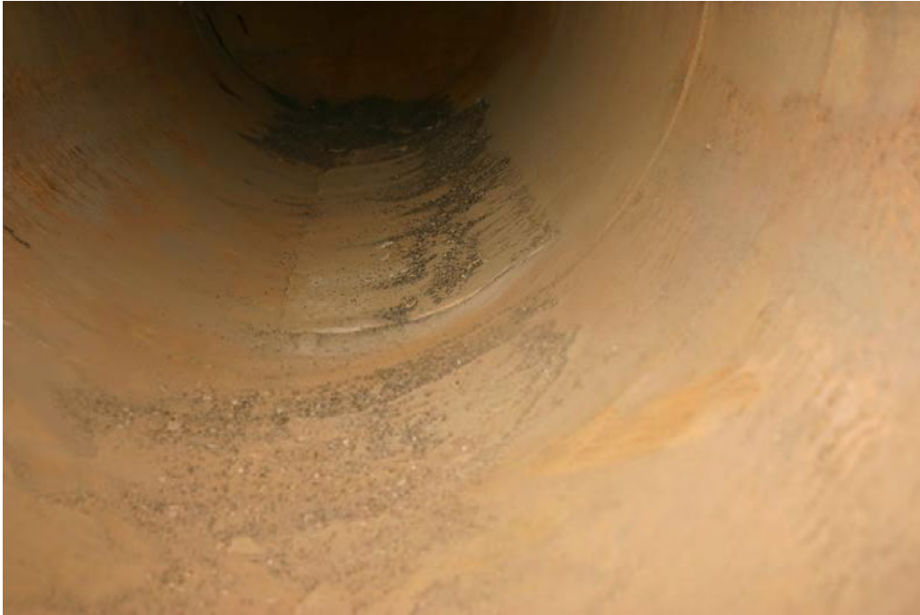
Photograph 9 – Poorly adhering thick-film coating inside the 32” nozzle at about the 35’ to 45’ stations
