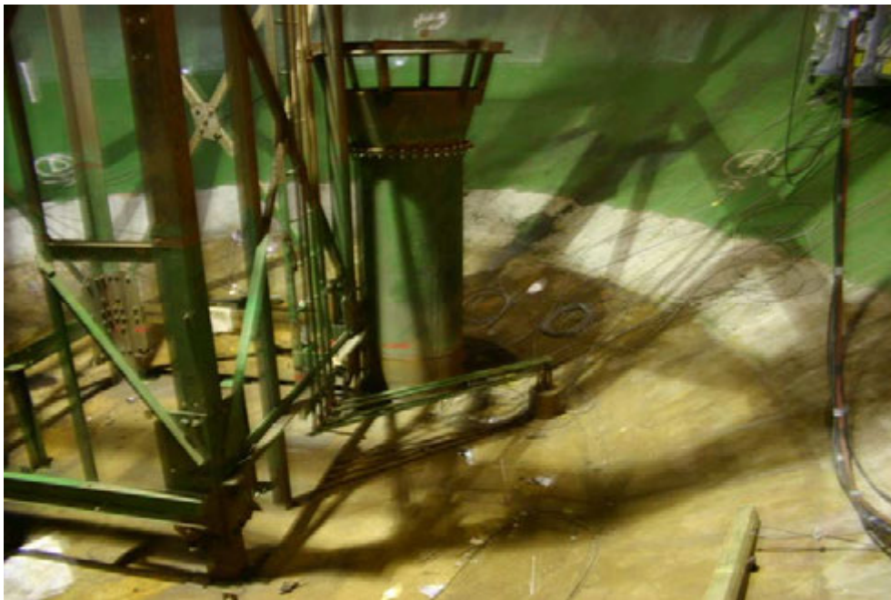
Photograph 12 – Bottom of the tank. Note the 32-inch inlet/outlet line and the 4 x \frac{3}{4} -inch sample lines.
