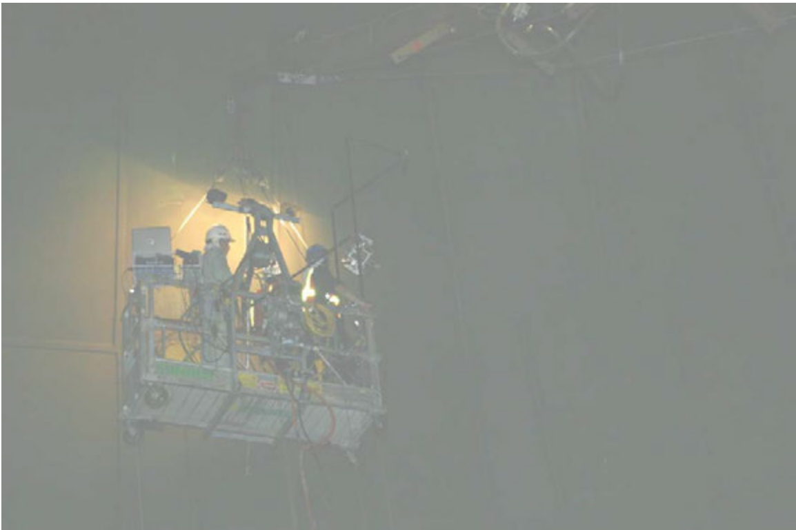
Inspection team #1 using the Viper LFET/U.T. Crawler on course C in Quadrant C of the Upper Dome.
