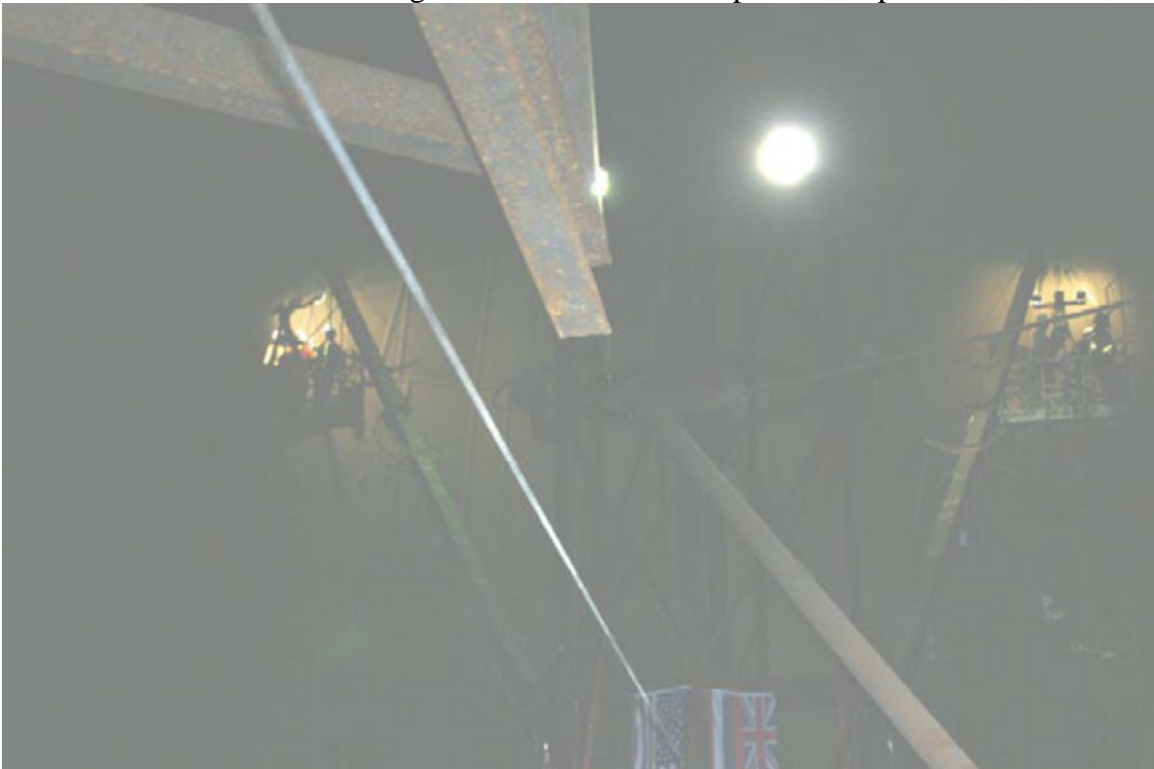
Both inspection crews in the Upper Dome during Viper LFET/U.T. Crawler work.
