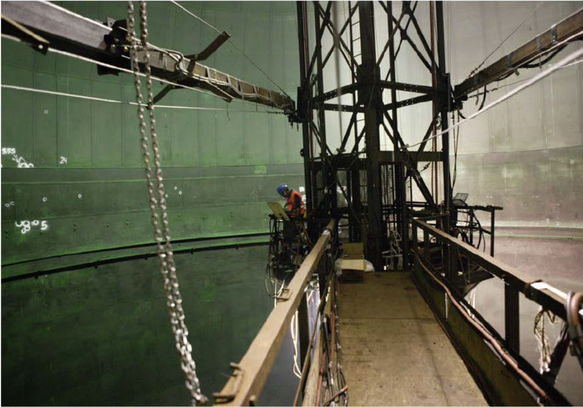
The catwalk, tower, and tank interior viewed looking in from the manway.
