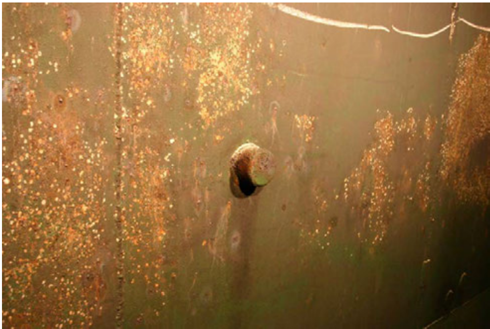
Photograph 6 – A 3-inch grout nozzle that has not been examined by UT testing or eddy current scanning.
