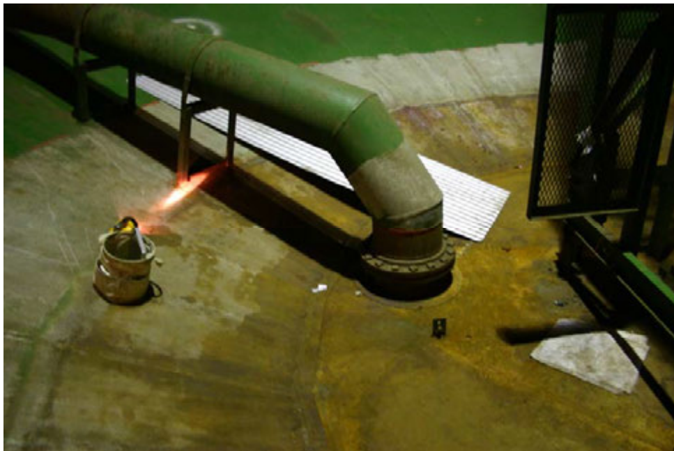
Photograph 8 – The 18-inch inlet/outlet line.
