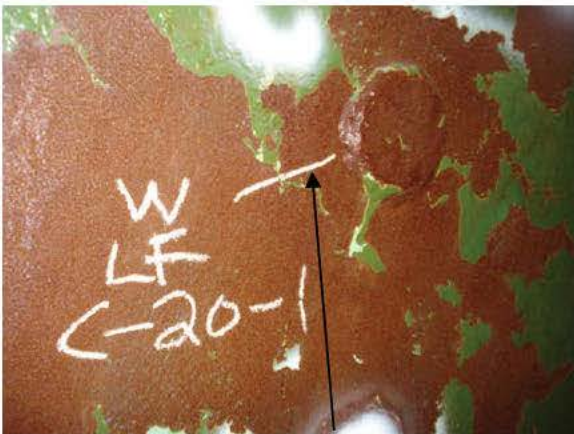
C-P20-1 WELD REPAIR- LACK OF FUSION
