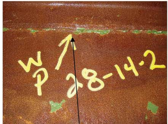
R28-P14-2 WELD REPAIR- POROSITY
