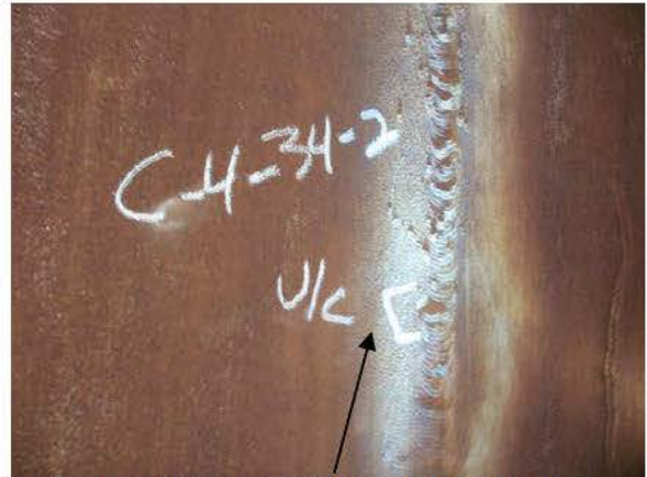
C4-P34-2 WELD REPAIR- UNDERCUT
