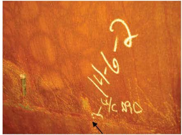
R14-6-2 WELD REPAIR- UNDERCUT
