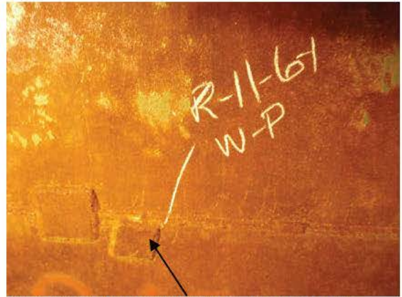
R11-P6-1 WELD REPAIR- POROSITY
