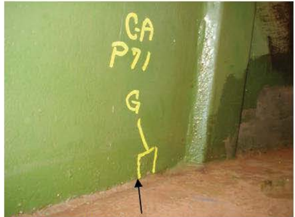
A-P71-3 GOUGE REPAIR
