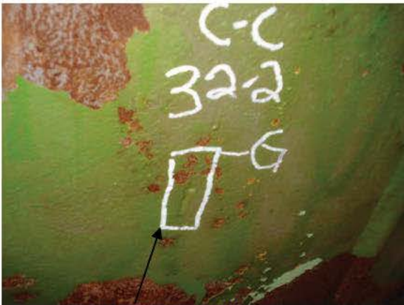
C-P32-2 GOUGE REPAIR
