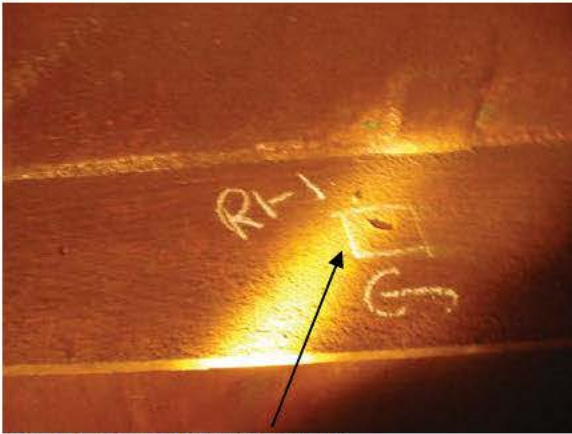
R1-P1-1 GOUGE REPAIR
