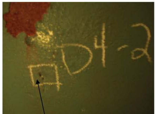
D-P4-2 GOUGE REPAIR
