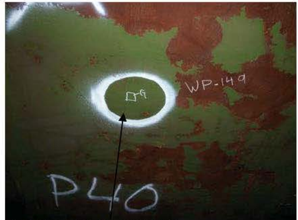
C-P40-2 GOUGE REPAIR
