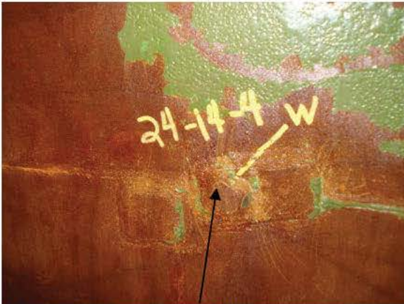
R24-P14-1 WELD REPAIR- LACK OF FUSION
