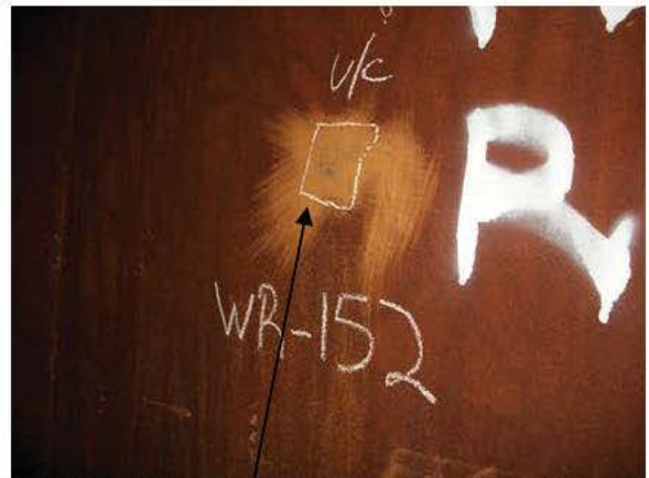
C4-P34-3 WELD REPAIR- UNDERCUT
