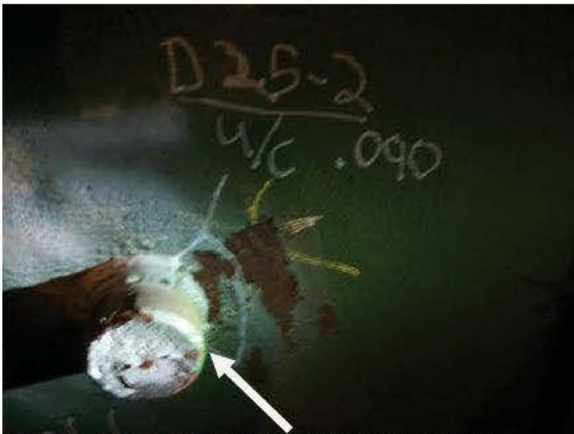
D-P25-2 WELD REPAIR-UNDERCUT
