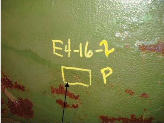
E4-P16-2 PIT REPAIR
