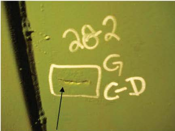
D-P28-2 GOUGE REPAIR
