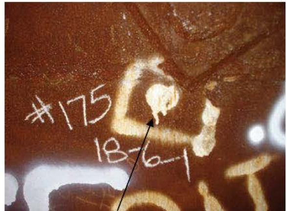
R18-P6-1 GOUGE REPAIR
