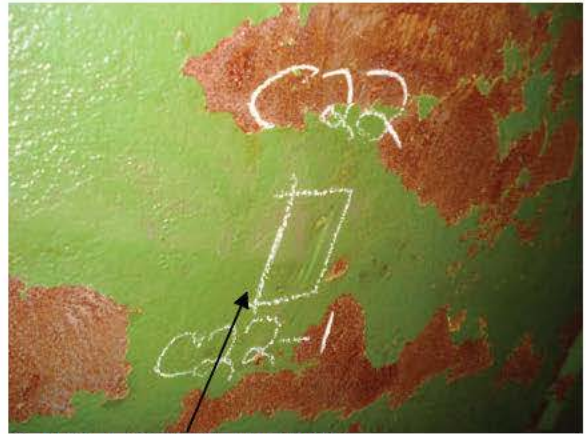
C-P22-1 GOUGE REPAIR
