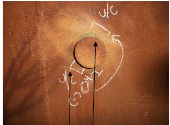
C3-P34-1 WELD REPAIR- UNDERCUT
