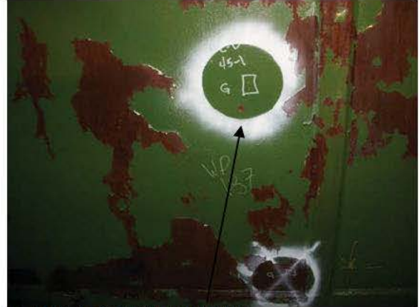
D-P45-1 GOUGE REPAIR
