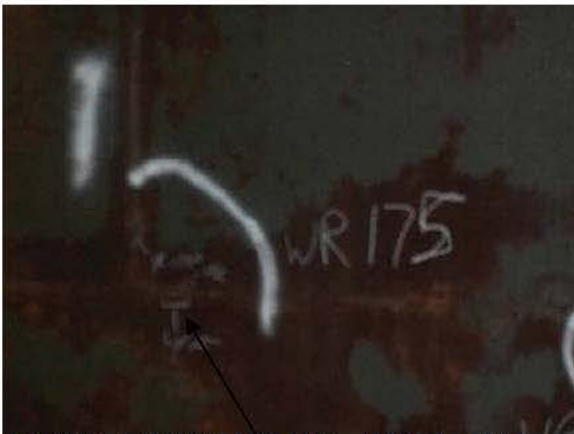
R6-P1P-1 WELD REPAIR- UNDERCUT
