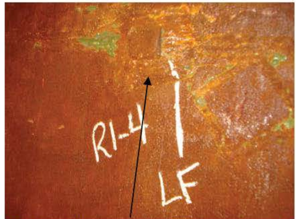
R1-P4-2 WELD REPAIR- LACK OF FUSION
