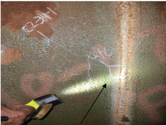
C2-P34-1 WELD- UNDERCUT
