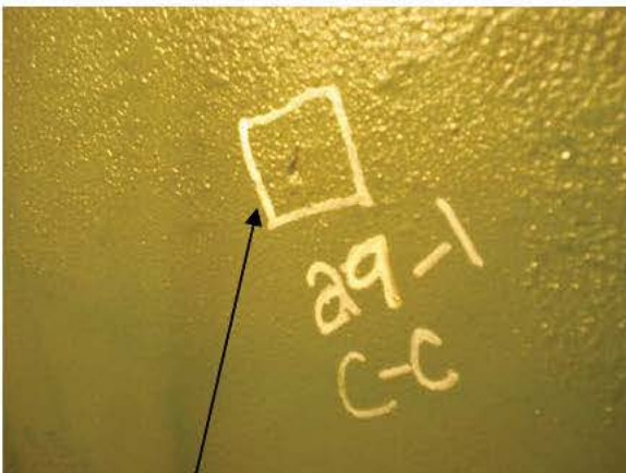
C-P29-1 GOUGE REPAIR
