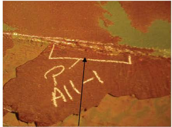
A-P11-1 WELD- POROSITY
