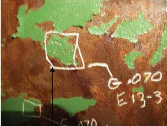
E-P13-3 GOUGE REPAIR
