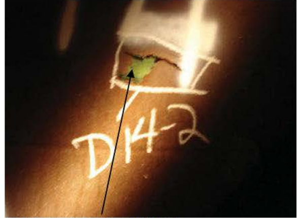
D-P14-2 GOUGE REPAIR
