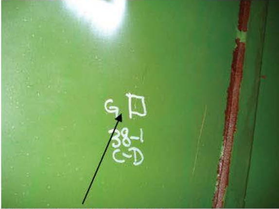
D-P38-1 GOUGE REPAIR
