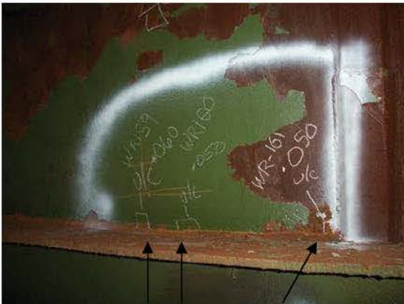
A-P37-1 WELD REPAIR- UNDERCUT
