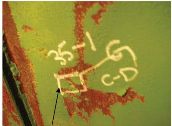
D-P35-1 GOUGE REPAIR
