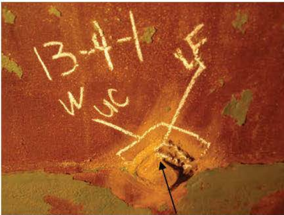
R13-P4-1 WELD REPAIR- LACK OF FUSION
