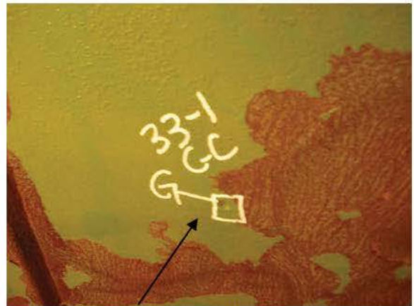
C-P33-1 GOUGE REPAIR
