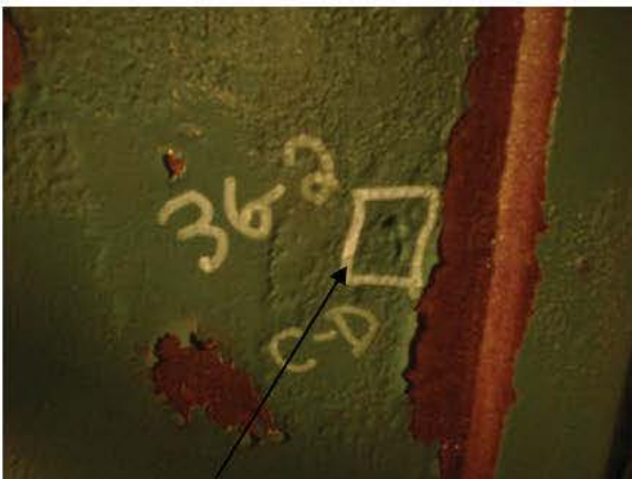
D-P36-2 GOUGE REPAIR
