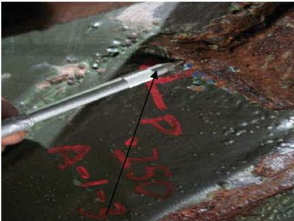
A-P1-3 WELD REPAIR- UNDERCUT
