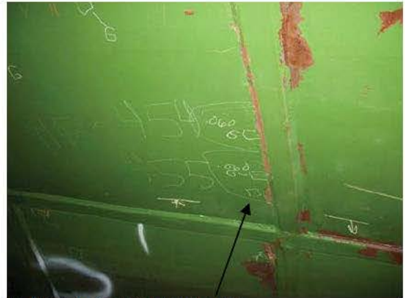
D-P26-1 GOUGE REPAIR
