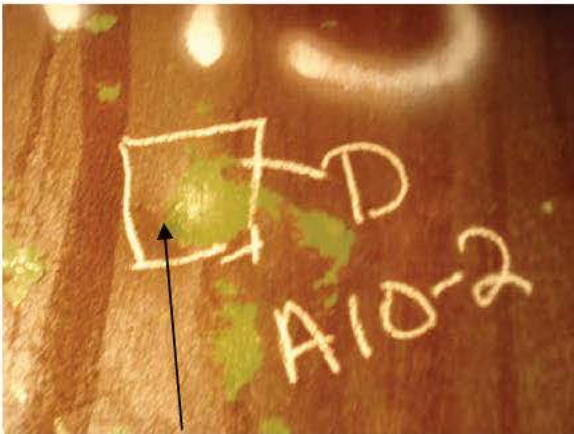
A-P10-2 DENT REPAIR
