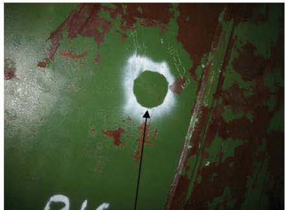
D-P16-2 GOUGE REPAIR
