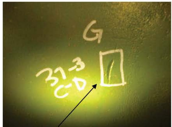
D-P37-3 GOUGE REPAIR
