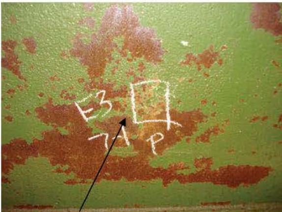
E3-P7-1 PIT REPAIR
