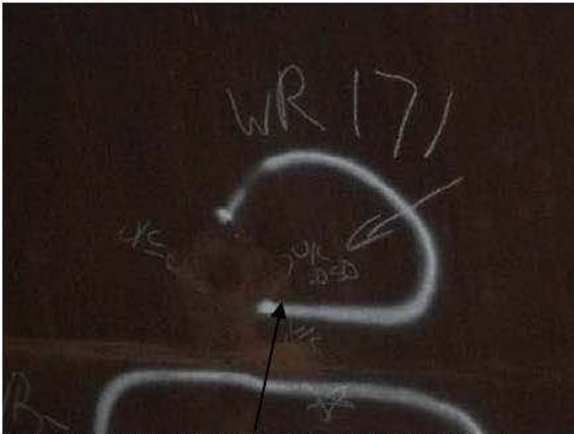
C4-P1-1 WELD REPAIR- UNDERCUT
