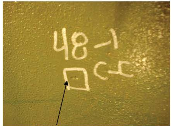
C-P48-1 GOUGE REPAIR
