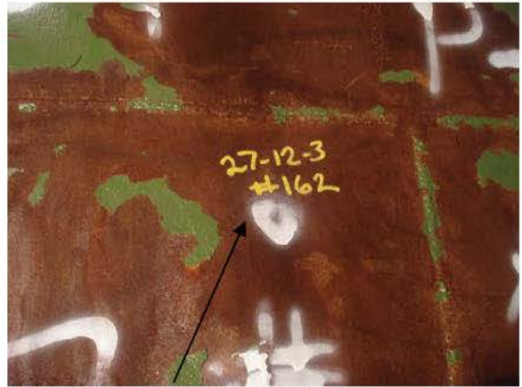
R27-P12-3 GOUGE REPAIR
