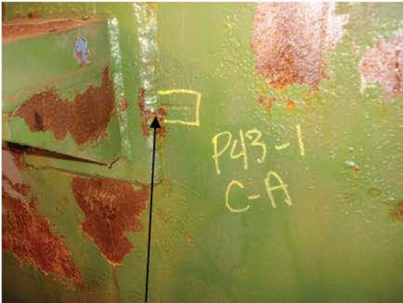
A-P43-1 GOUGE REPAIR
