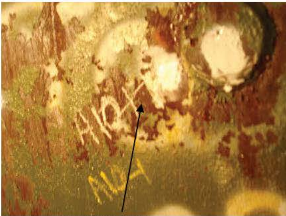
A-P10-1 DENT REPAIR
