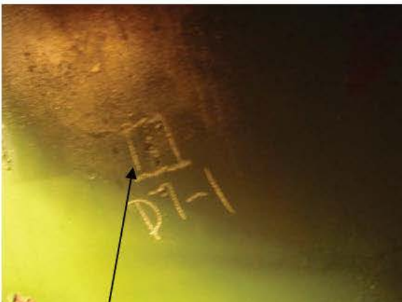
D-P7-1 GOUGE REPAIR
