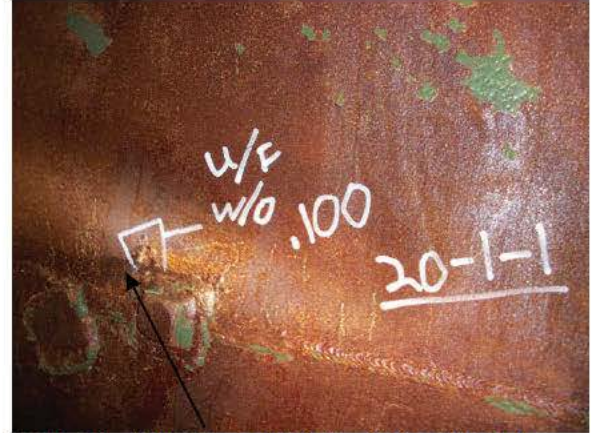
R20-P1-1 WELD REPAIR- UNDERFILL
