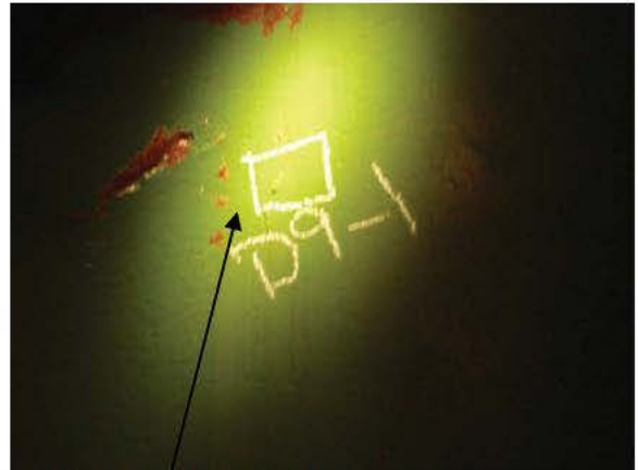
D-P9-1 GOUGE REPAIR
