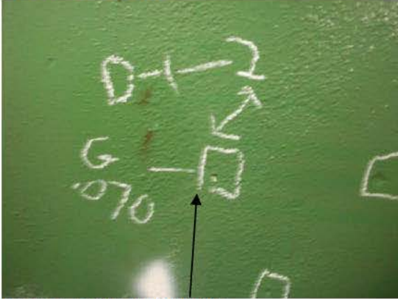
D-P1-2 GOUGE REPAIR
