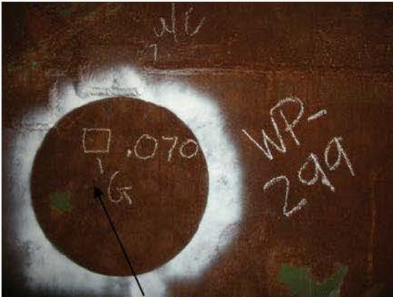
R10-P8-2 GOUGE REPAIR
