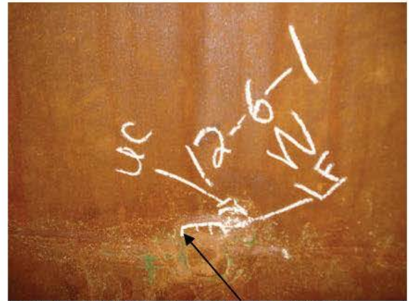
R12-P6-1 WELD REPAIR- LACK OF FUSION
