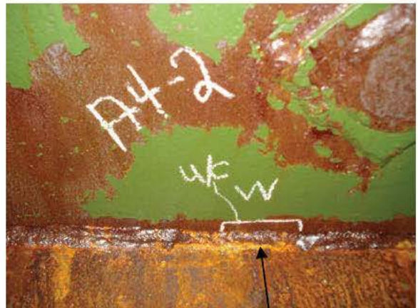
A-P4-2 WELD REPAIR - UNDERCUT
