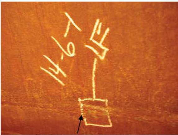
R14-P6-1 WELD REPAIR- LACK OF FUSION
