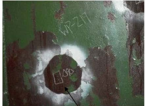
D-P19-2 GOUGE REPAIR
