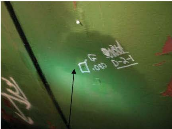
D-P2-1 GOUGE REPAIR
