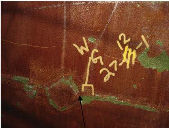
R27-P12-1 GOUGE REPAIR
