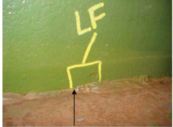
A-P71-2 WELD REPAIR- LACK OF FUSION
