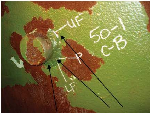
B-P50-1 WELD REPAIR- LACK OF FUSION POROSITY UNDERFILL
