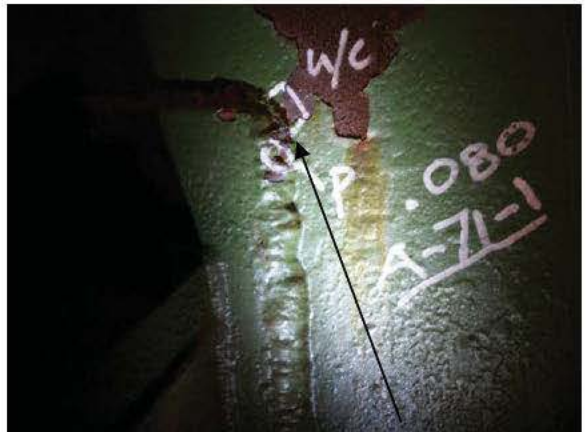
A-P71-1 WELD REPAIR- UNDERCUT
