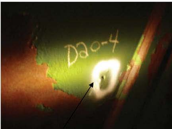
D-P20-4 GOUGE REPAIR
