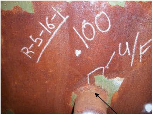
R5-P16-1 WELD REPAIR- UNDERFILL
