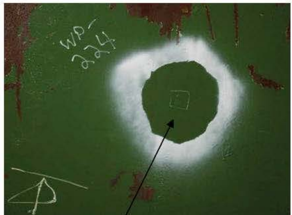
D-P11-1 GOUGE REPAIR
