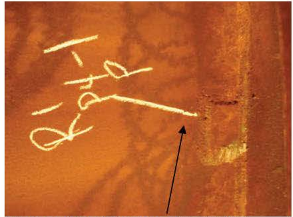
R1-P4-1 WELD REPAIR- POROSITY
