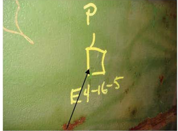
E4-P16-5 PIT REPAIR
