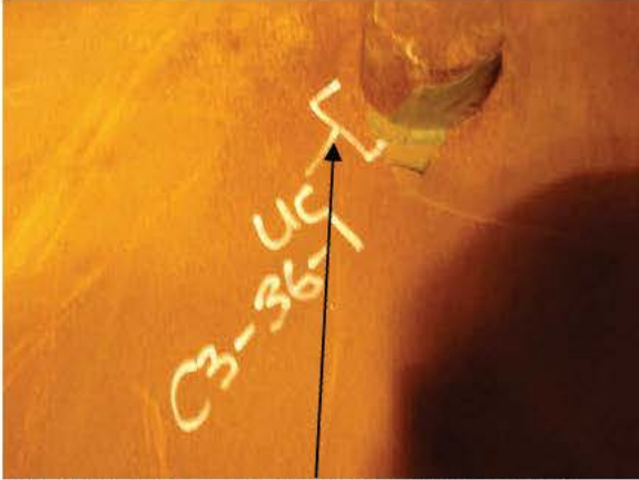
C3-P36-1 WELD REPAIR- UNDERCUT
