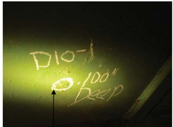
D-P10-1 GOUGE REPAIR
