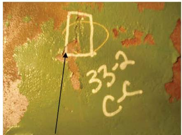
C-P33-2 GOUGE REPAIR
