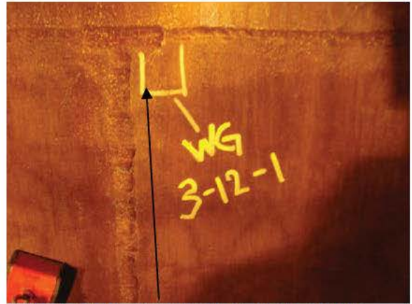
R3-P12-1 WELD REPAIR- POROSITY
