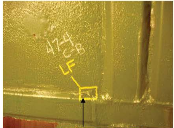
B-P47-4 WELD REPAIR- LACK OF FUSION
