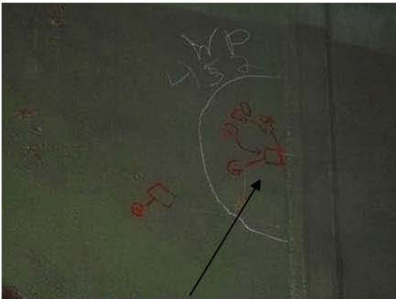
C-1-1 GOUGE REPAIR
