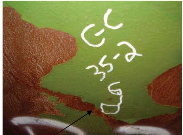
C-P35-2 GOUGE REPAIR
