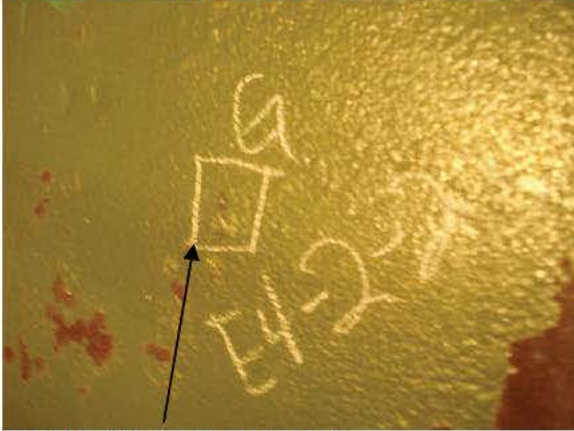
E4-P2-2 GOUGE REPAIR
