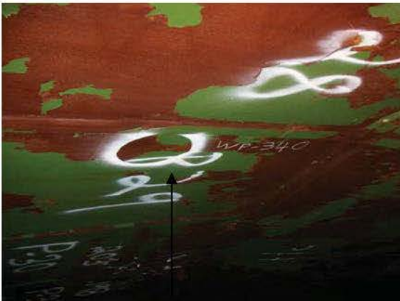
D-P29-1 GOUGE REPAIR
