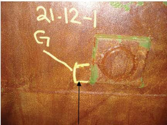
R21-P12-1 GOUGE REPAIR
