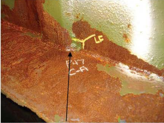
A-P47-1 WELD REPAIR- LACK OF FUSION
