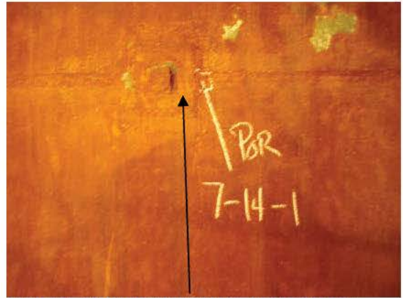
R7-P14-1 WELD REPAIR- POROSITY
