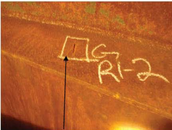
R1-P2-1 GOUGE REPAIR
