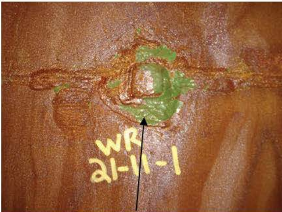
R21-P11-1 EXCESS WELD REINFORCEMENT
