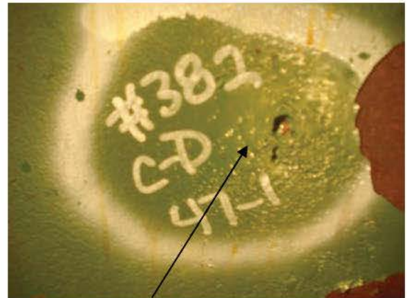
D-P47-1 GOUGE REPAIR
