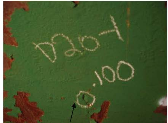
D-P20-1 GOUGE REPAIR
