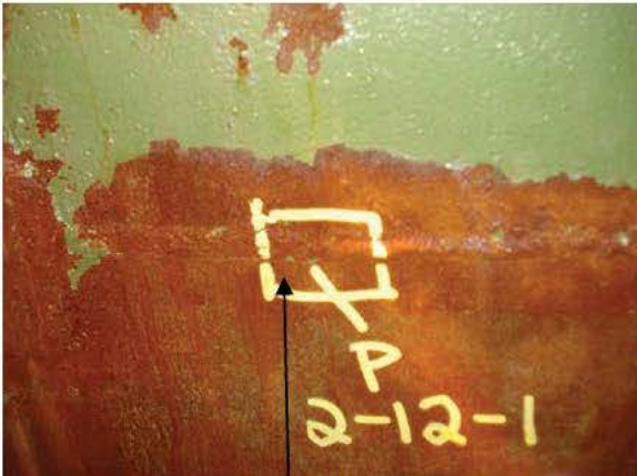
R2-P12-1 WELD REPAIR- POROSITY
