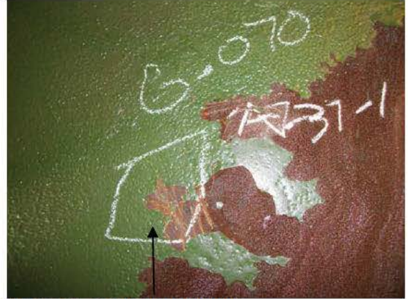
A-P37-2 GOUGE REPAIR
