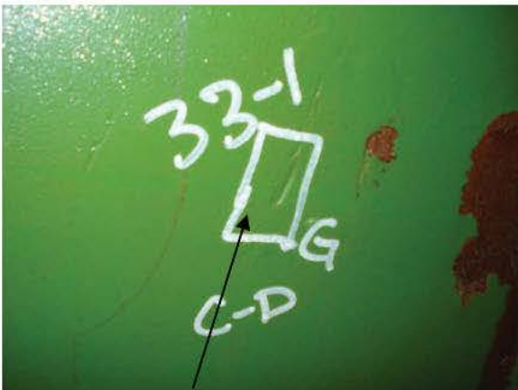
D-P33-1 GOUGE REPAIR
