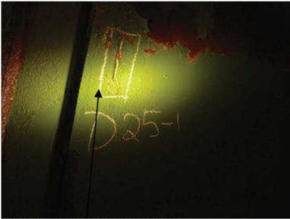
D-P25-1 GOUGE REPAIR
