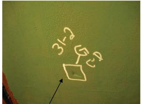
D-P31-2 GOUGE REPAIR
