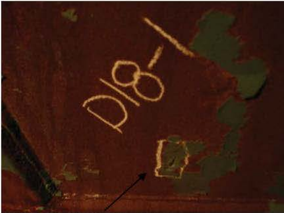
D-P18-1 GOUGE REPAIR
