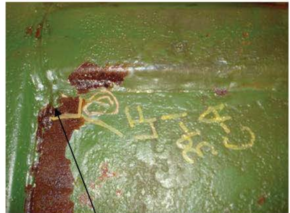
A-P39-1 WELD REPAIR- LACK OF FUSION
