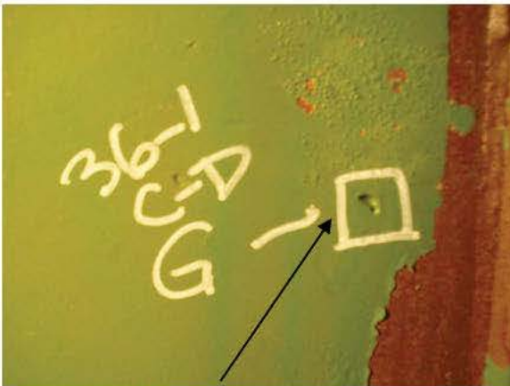
D-P36-1 GOUGE REPAIR
