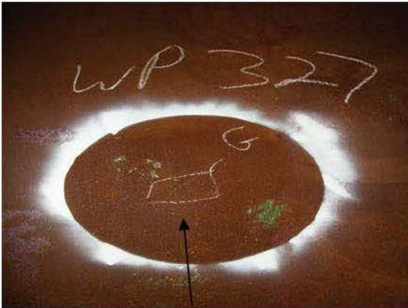
R26-P8-1 GOUGE REPAIR
