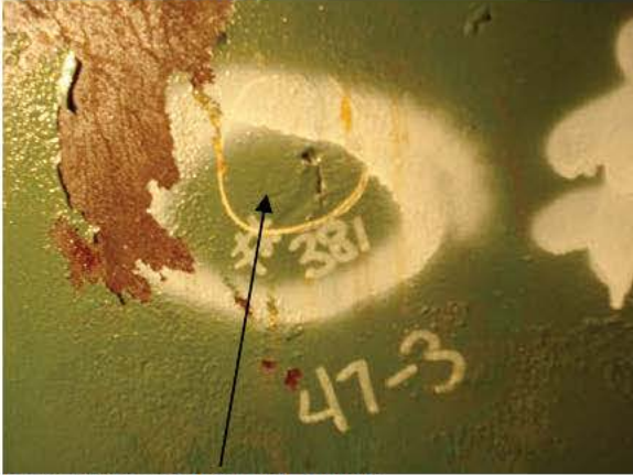
D-P47-3 GOUGE REPAIR
