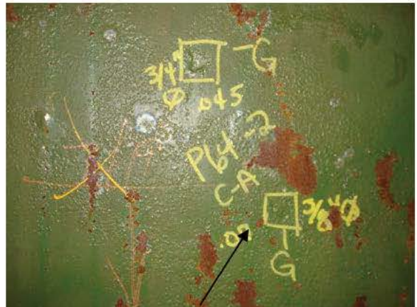
A-P64-2 GOUGE REPAIR
