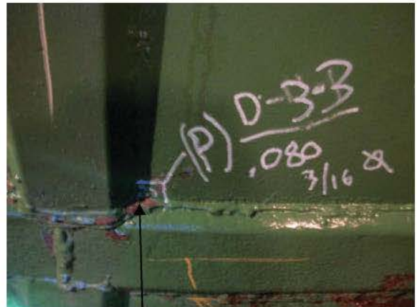
D-P3-3 GOUGE REPAIR
