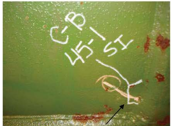
B-P45-1 WELD REPAIR- SLAG INCLUSION
