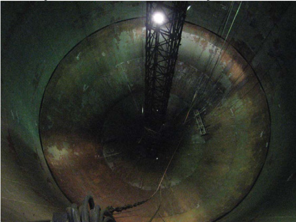
Lower dome view from above showing extensive coating failure.
