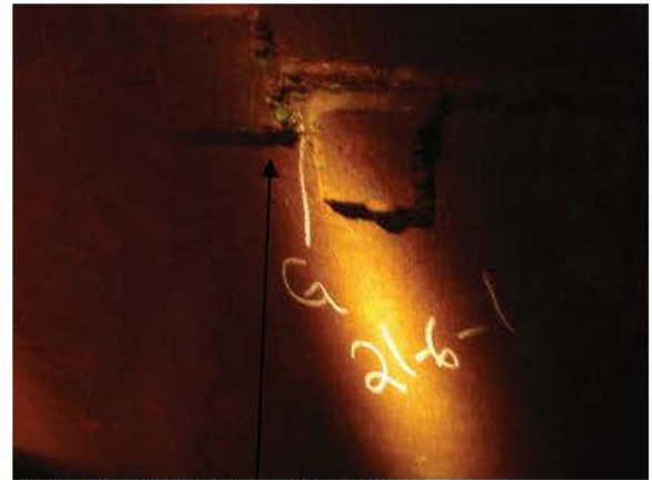
R21-P6-1 GOUGE REPAIR
