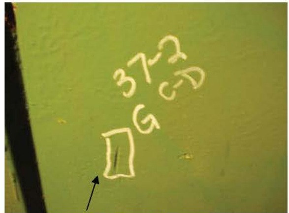
D-P37-2 GOUGE REPAIR
