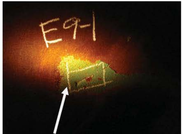
E-P9-1 GOUGE REPAIR
