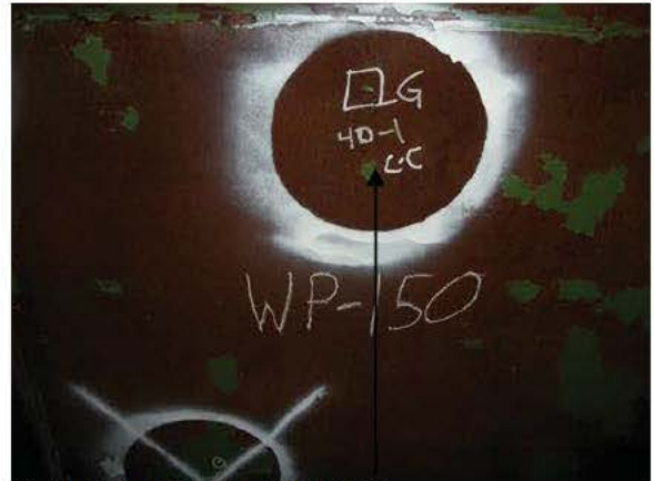
C-P40-1 GOUGE REPAIR
