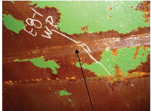
E-P8-1 WELD REPAIR- POROSITY
