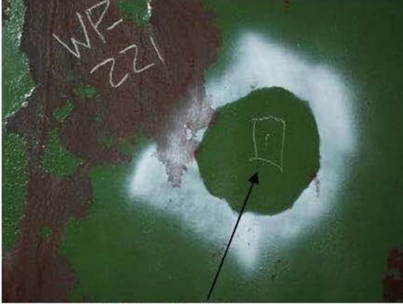
D-P17-1 GOUGE REPAIR
