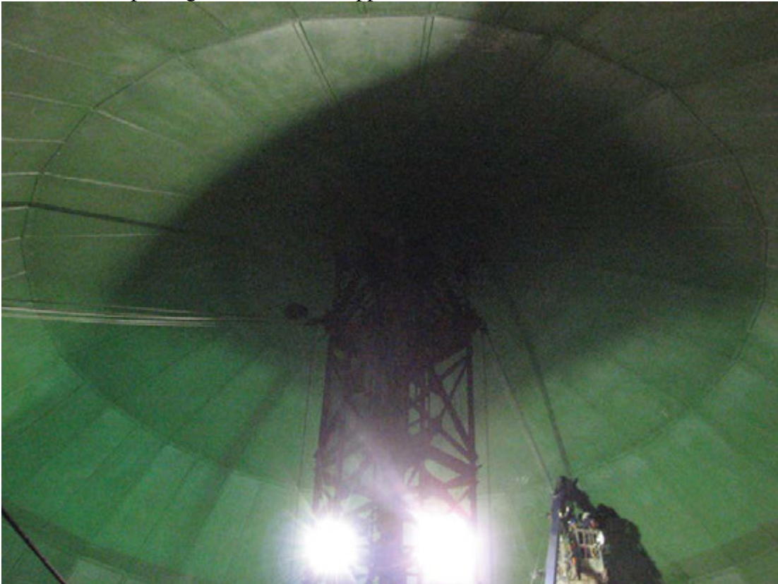
A view of the very top of tank (Typical Tank upper dome section)
