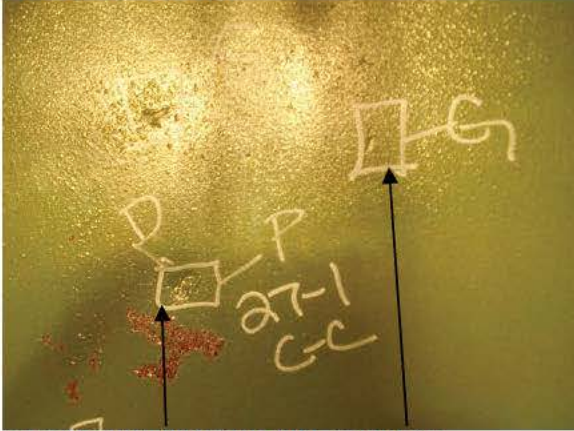
C-P27-1 DENT REPAIR, GOUGE
