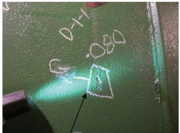
D-P1-1 GOUGE REPAIR
