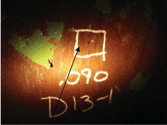
D-P13-1 GOUGE REPAIR
