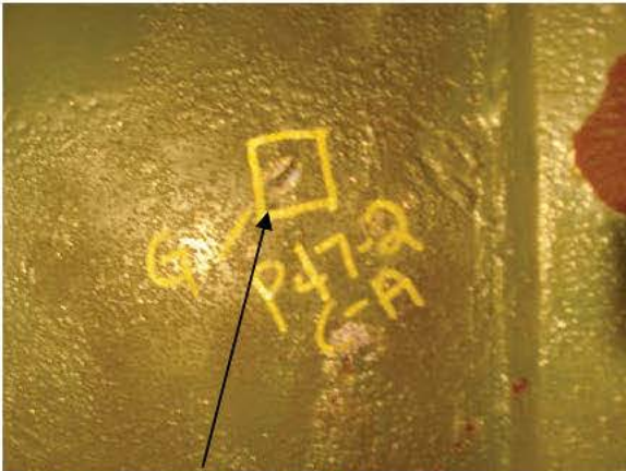
A-P47-2 GOUGE REPAIR
