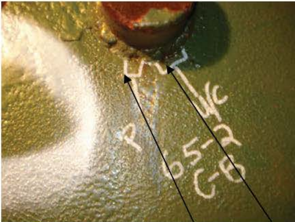
B-P65-2 WELD REPAIR- POROSITY, UNDERCUT
