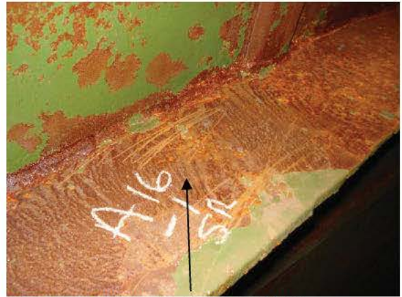
A-P16-1 MULTIPLE PIT REPAIR
