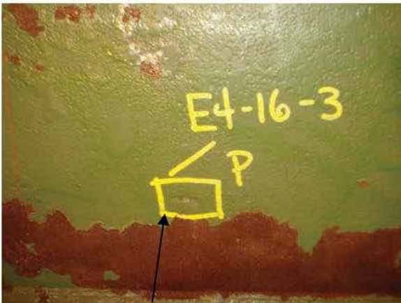
E4-P16-3 PIT REPAIR
