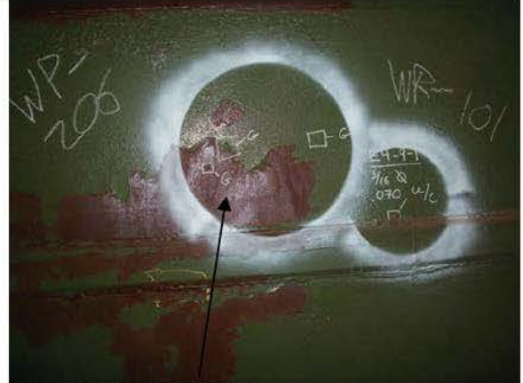
E4-P9-2 PIT REPAIR
