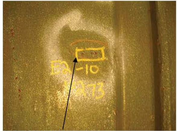
E2-P10-1 PIT REPAIR
