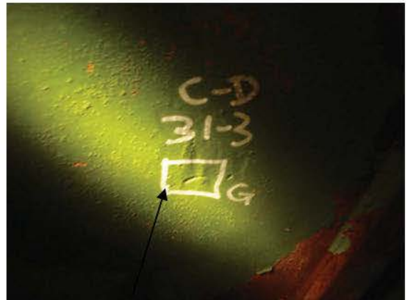
D-P31-3 GOUGE REPAIR
