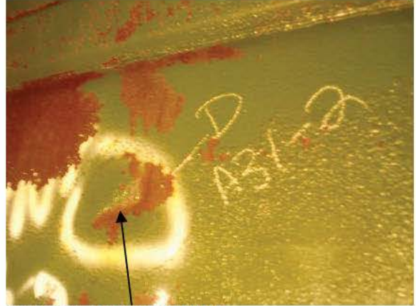
A-P31-2 DENT REPAIR
