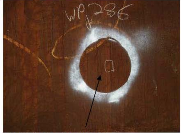
R2-P2-1 GOUGE REPAIR
