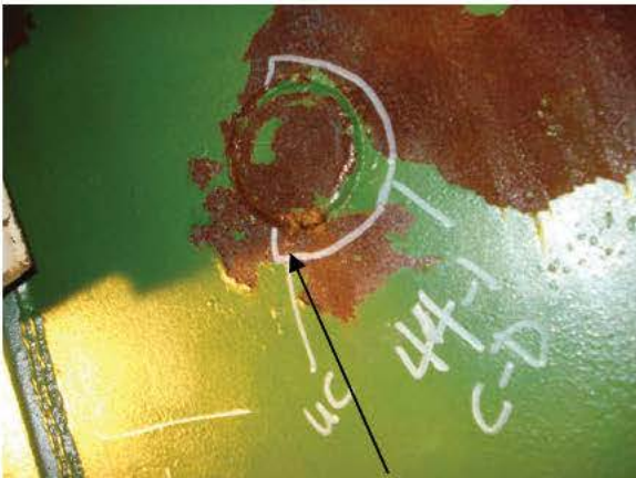
D-P44-1 WELD - UNDERCUT
