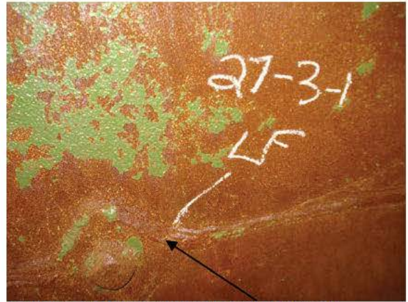
R27-P3-1 WELD REPAIR- LACK OF FUSION
