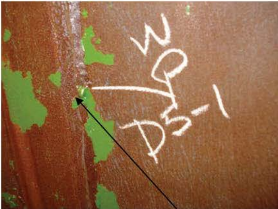
D-P5-1 WELD REPAIR- POROSITY
