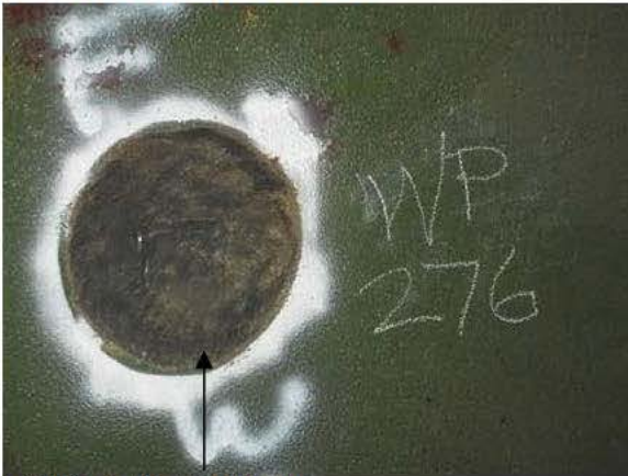
E2-P3-1 PIT REPAIR
