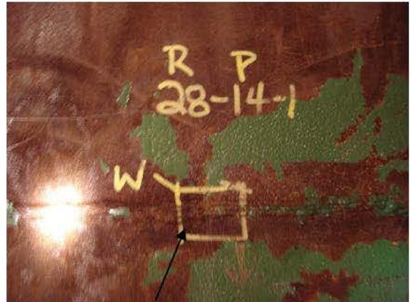
R28-P14-1 WELD REPAIR- LACK OF FUSION
