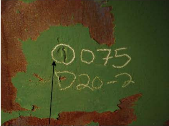
D-P20-2 GOUGE REPAIR
