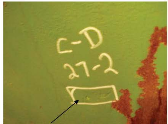
D-P27-2 GOUGE REPAIR
