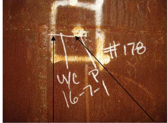
R16-P7-1 WELD REPAIR- UNDERCUT, POROSITY
