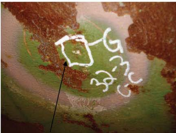
C-P32-4 GOUGE REPAIR
