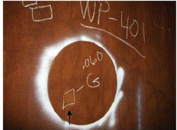
R11-P8-3 GOUGE REPAIR
