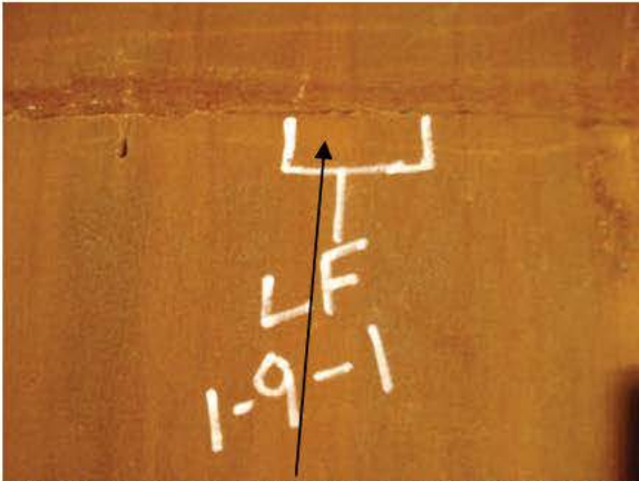
R1-P9-1 WELD REPAIR- LACK OF FUSION
