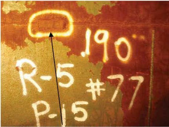
R5-P15-2 WELD REPAIR- UNDERFILL
