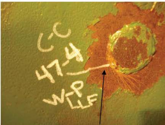
C-P47-4 WELD REPAIR- LACK OF FUSION
