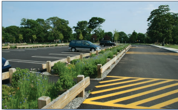
Figure 2. Project partners installed vegetated bioinfiltration swales in this parking lot near the beach.
