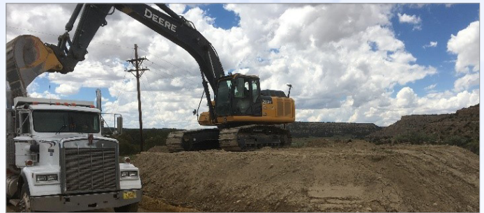
Arrow Indian Contractors, a USEPA contractor, removes 10,000 cubic yards of contaminated soil at the Quivira mine site.
