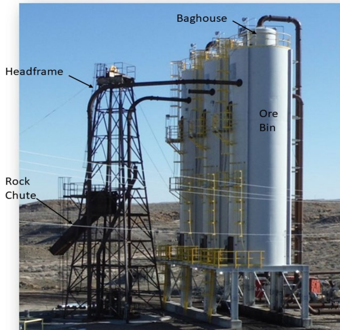
Photograph 1: Ore bins with baghouses adjacent to headframe
